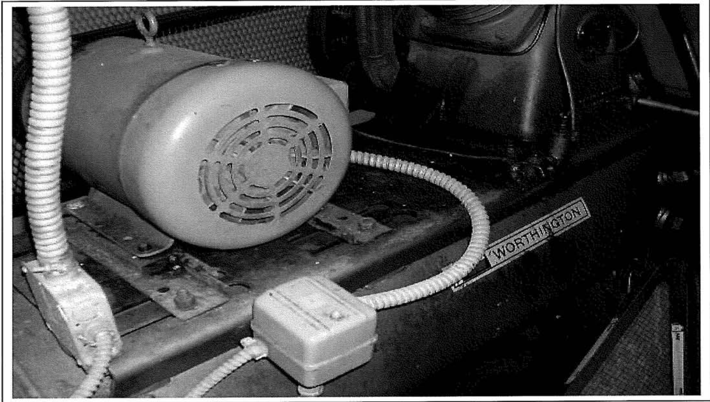
Photo 61: Floor mounted compressor in mechanical room adjacent nutrition area, Section 5, Therapy Building.
