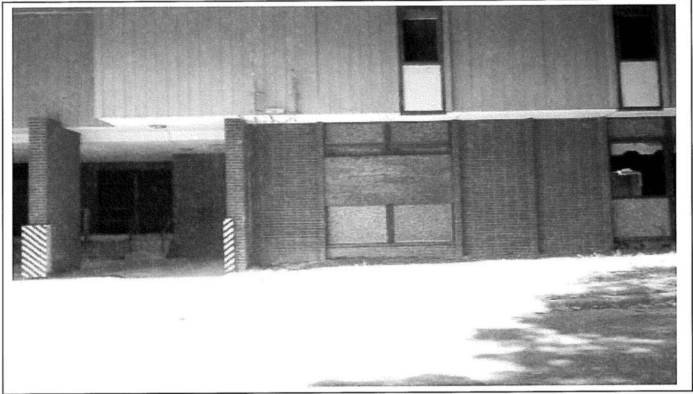
Photo 11: View of side elevation of cottage No. 3 depicting the brick/wood exterior façade.
