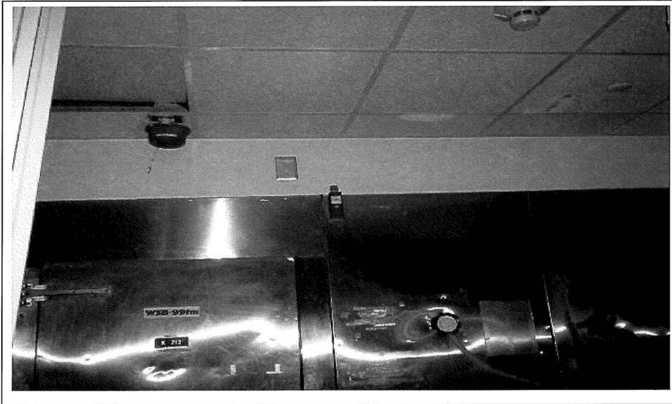
Photo 74: Typical wall-mounted coolers located in the storage area of section 6, Therapy building.
