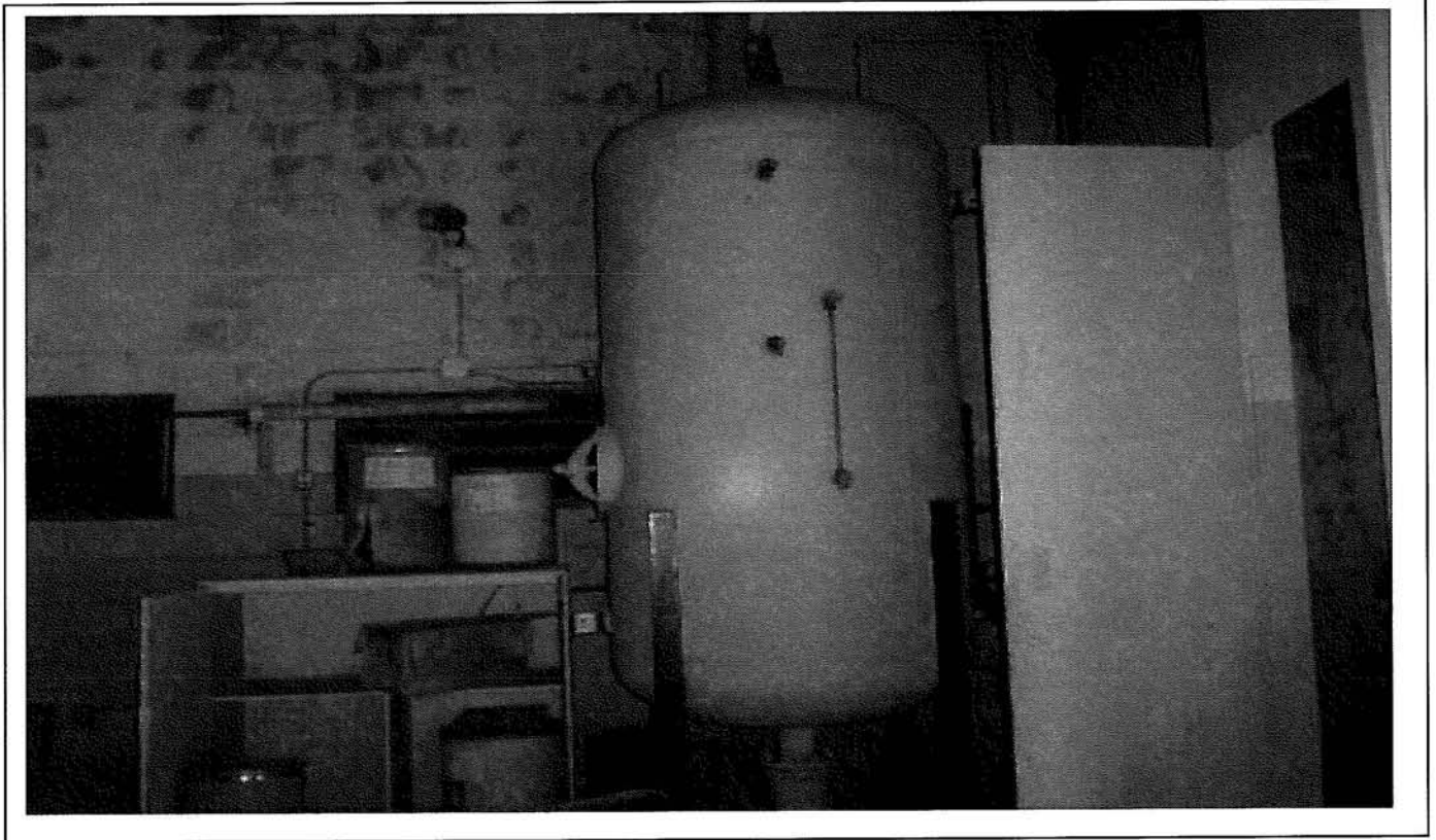
Photo 5: View of a chilled water storage tank in the power plant building.
