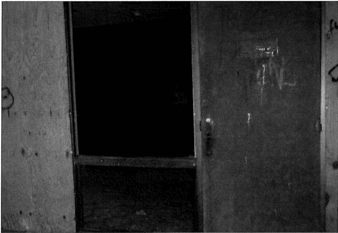
Photo 88: Typical Aluminum window framing located at the front entry of section 6, Therapy Building.
