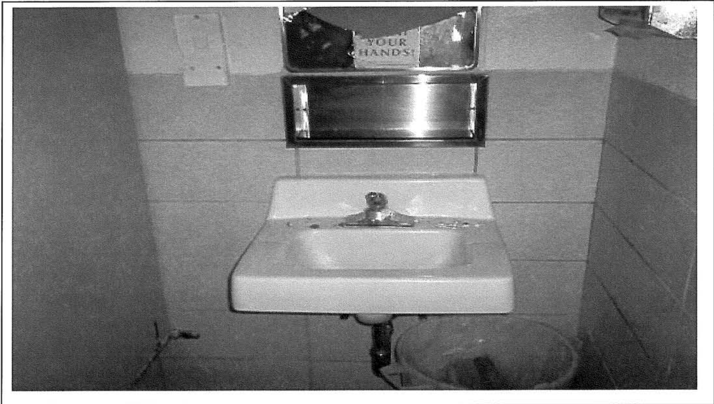
Photo 84: Typical ceramic sink located in locker area of section 6, Therapy Building.
