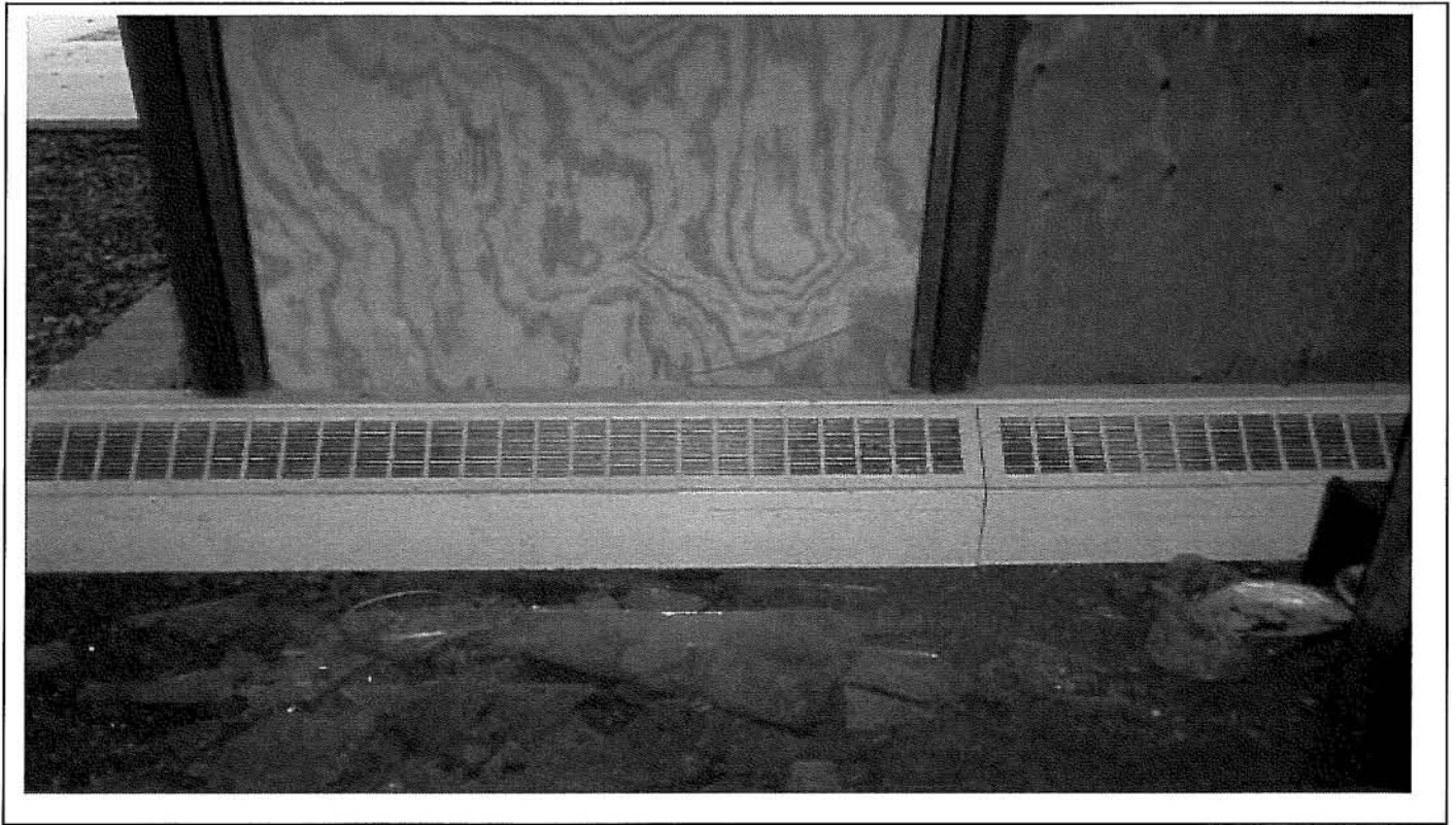
Photo 92: Typical floor-mounted heaters located in entryway of second floor section 5, Therapy Building.
