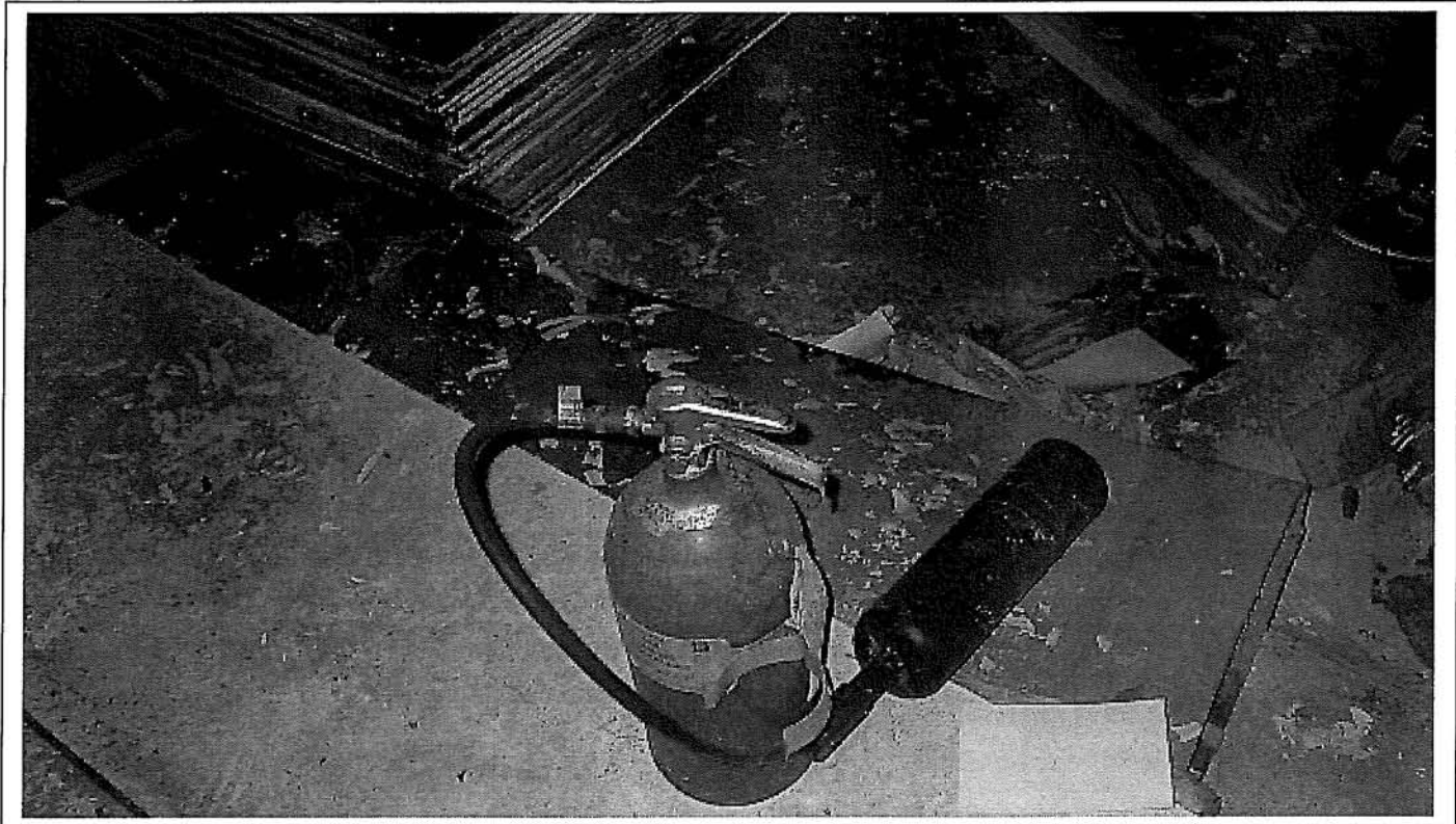
Photo 9: Typical fire extinguisher observed throughout property.
