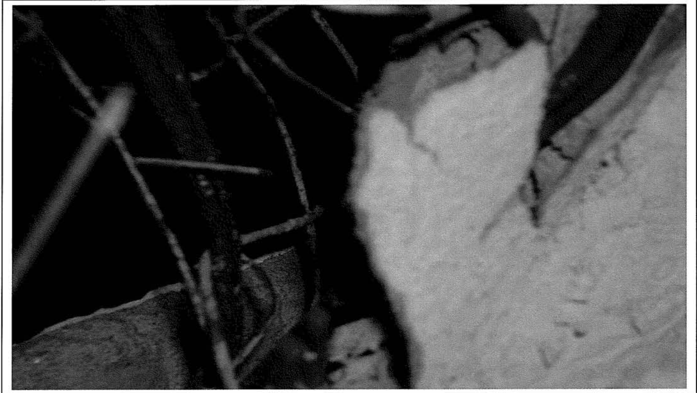
Photo 59: Typical view of metal re-enforcement in wall system of nutrition office area, Section 5, Therapy Building
