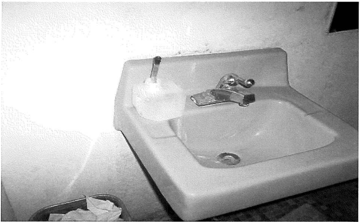
Photo 97: Typical blue ceramic sink located room on the ground floor, section 4 Therapy building.
