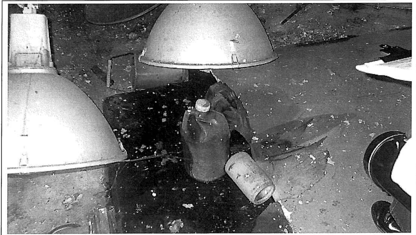
Photo 16: Oil leaking containers located in Power Plant.
