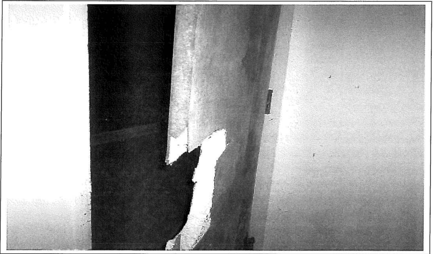
Photo 9: Typical Fire Door with Insulation containing ACM.
