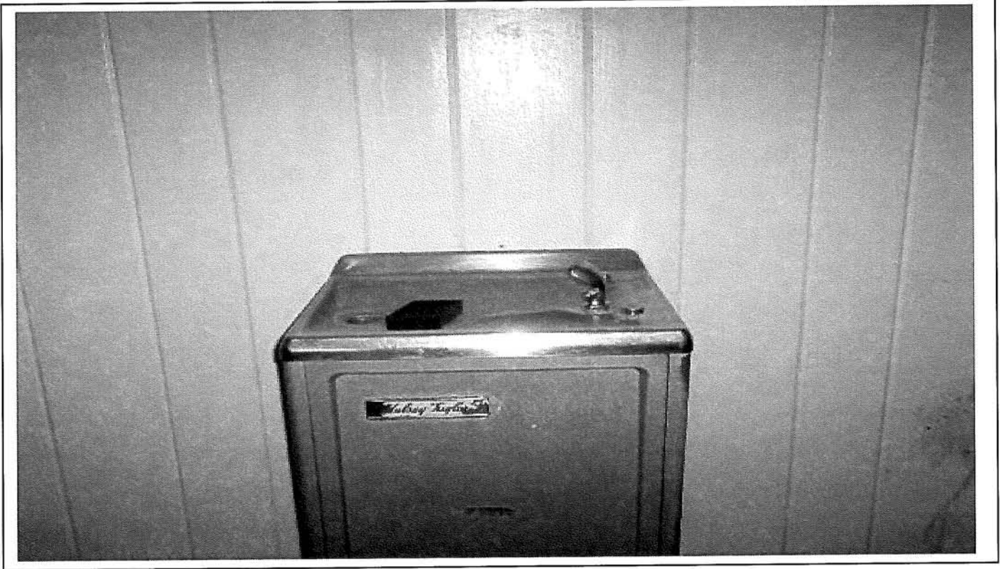
Photo 15: Typical metal, wall-mounted water fountain located in cottages.
