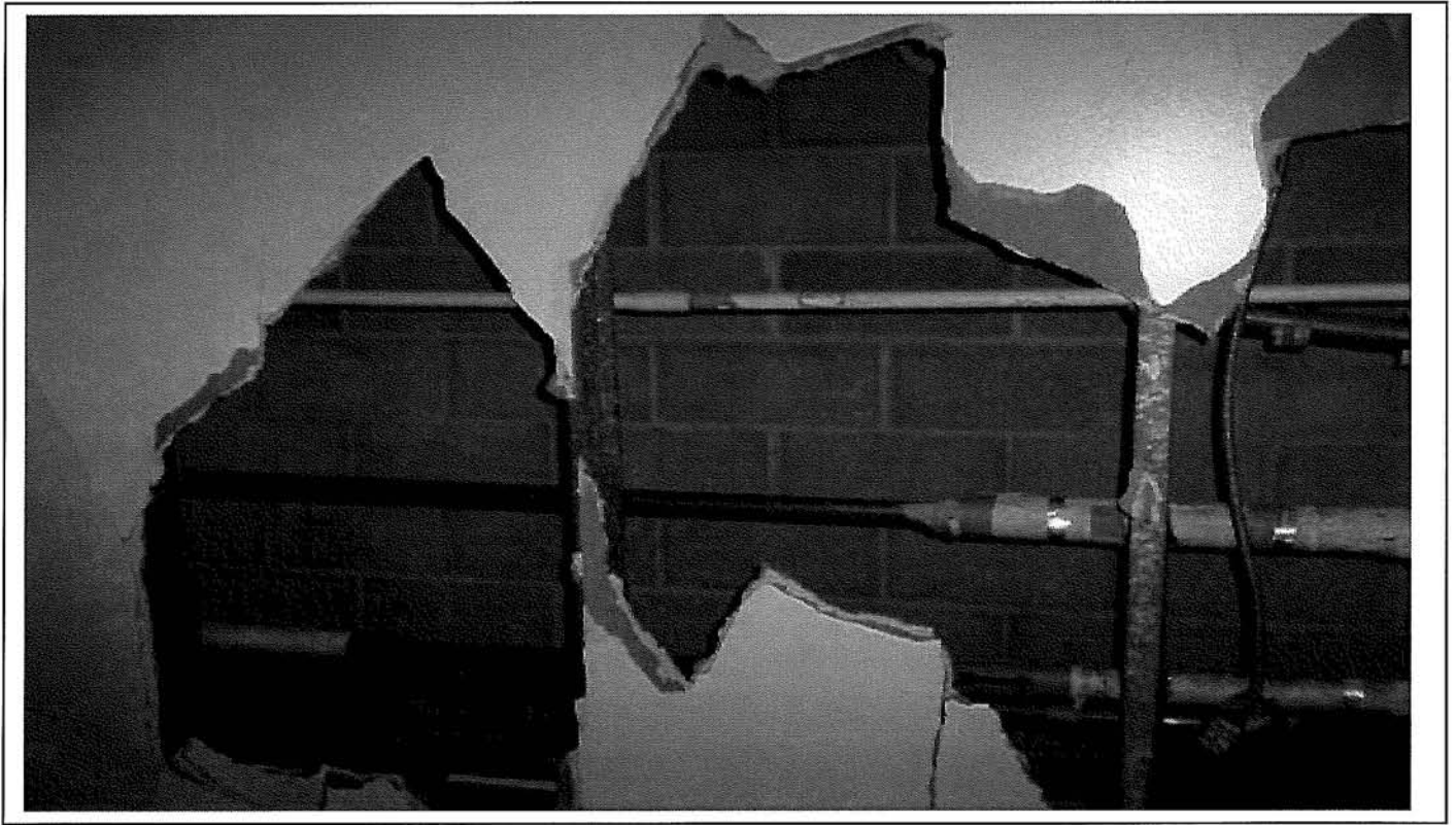
Photo 94: Typical copper tubing pipe run within pipe chase behind laboratory area on second floor section 5, Therapy Building.
