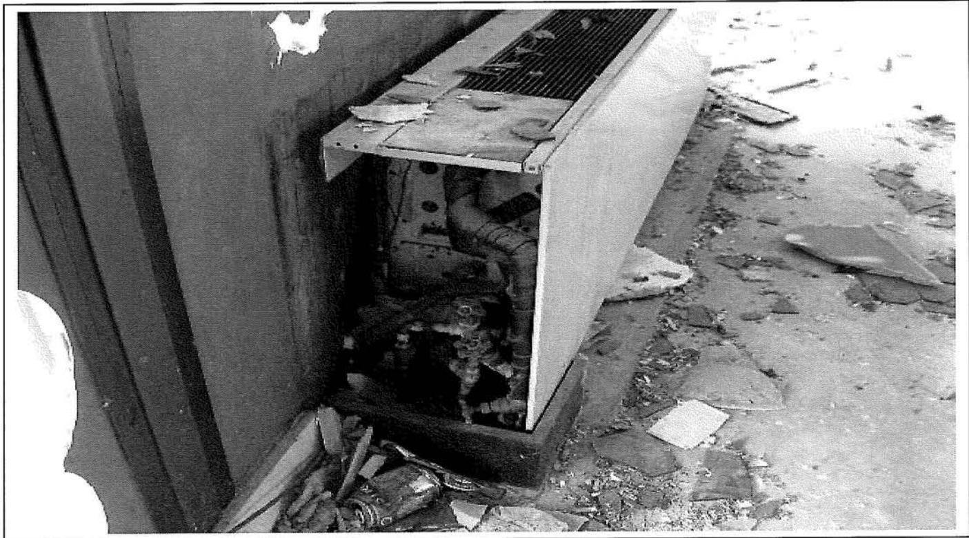
Photo 58: Typical wall-mounted radiator with copper piping in dining area Therapy Building.
