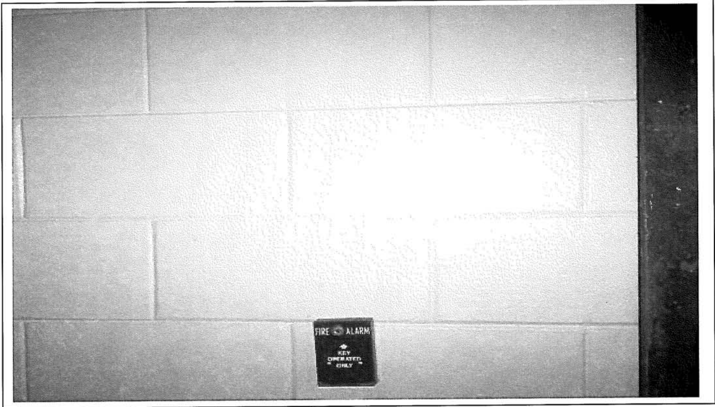
Photo 9: View of typical concrete masonry unit (CMU) system in lower level of cottage No. 3.
