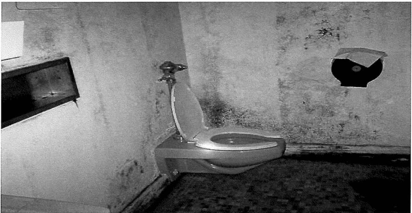
Photo 96: Typical toilet, blue ceramic material located room on the ground floor, section 4 Therapy building.
