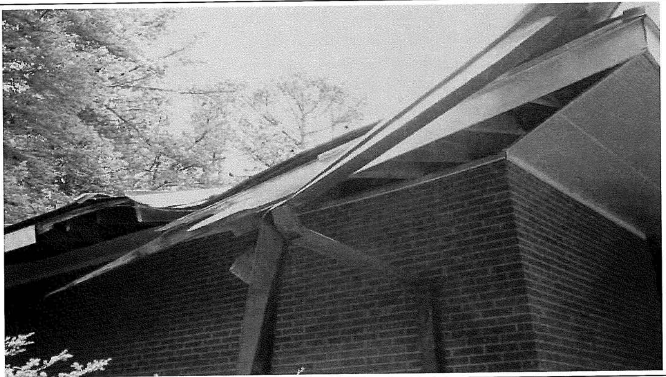
Photo 24: View of cottage No. 5 damage to roof section.
