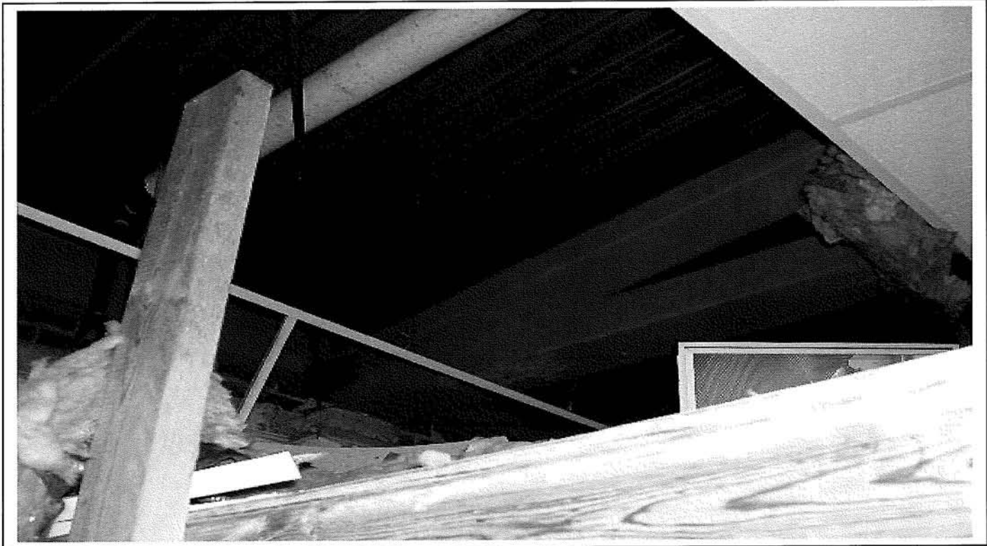
Photo 64: Typical coated metal beams, metal pan roof in , Section 5, of Therapy Building.
