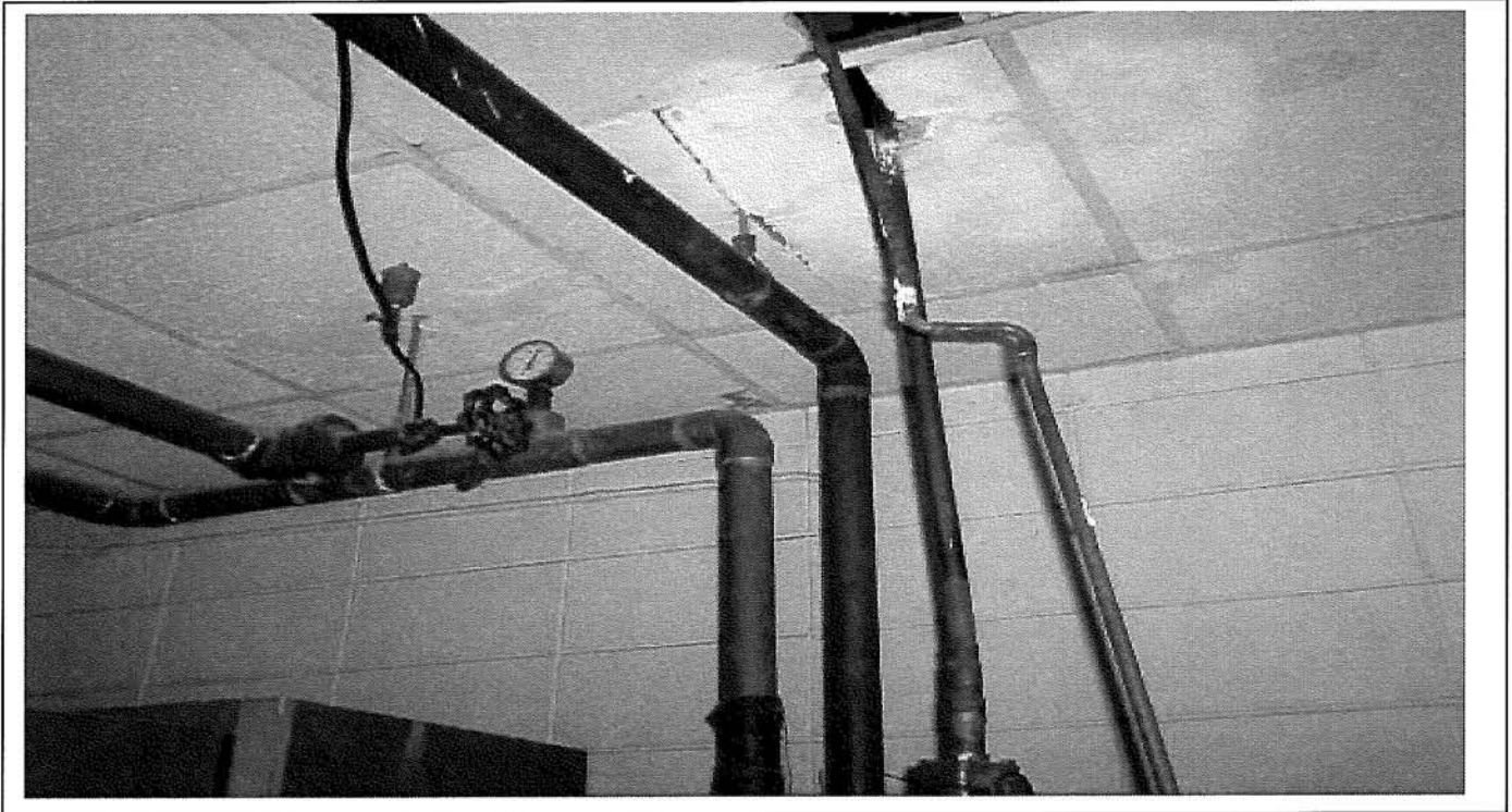
Photo 81: Typical copper pipe risers 2", 1" & ½" located in mechanical room of second level of section 6, Therapy Building.
