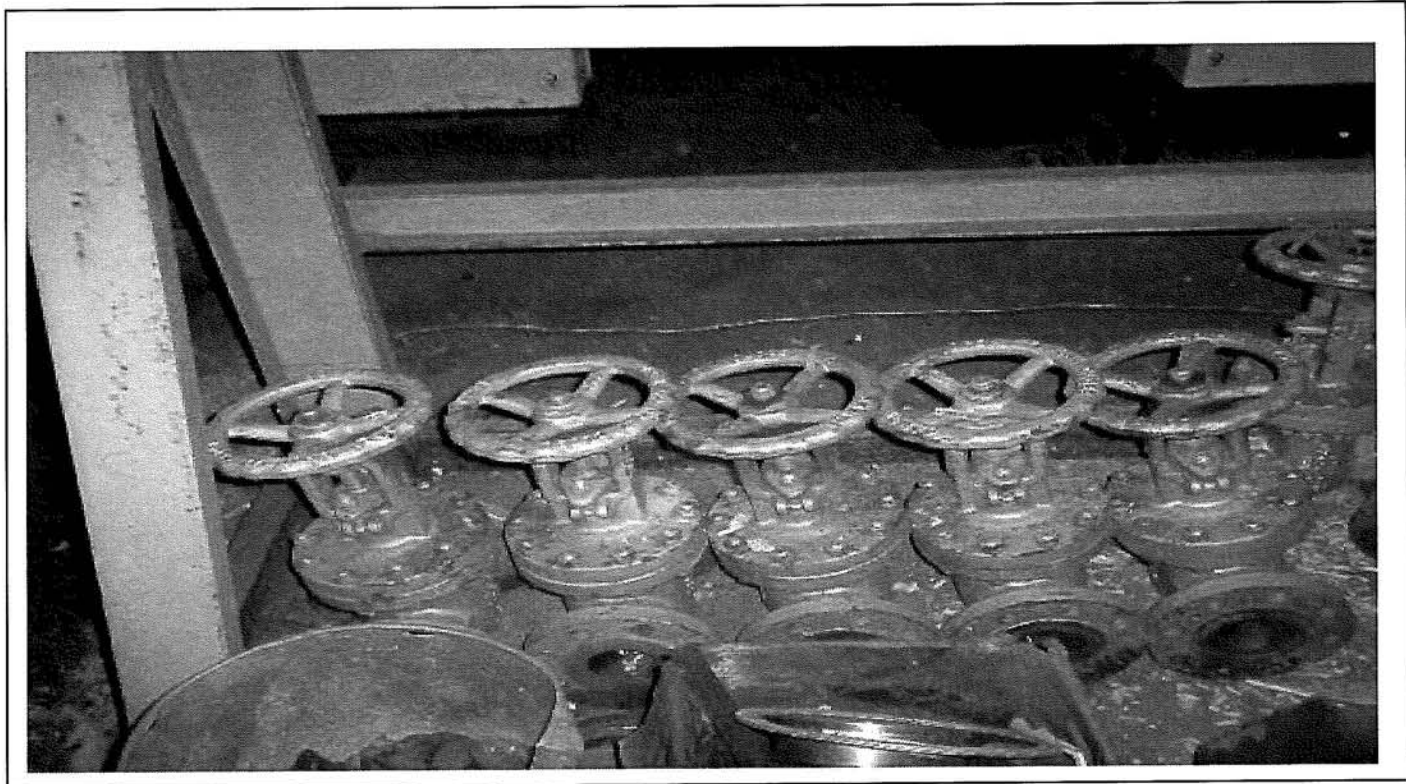
Photo 4: View of miscellaneous valves stored in the power plant building.
