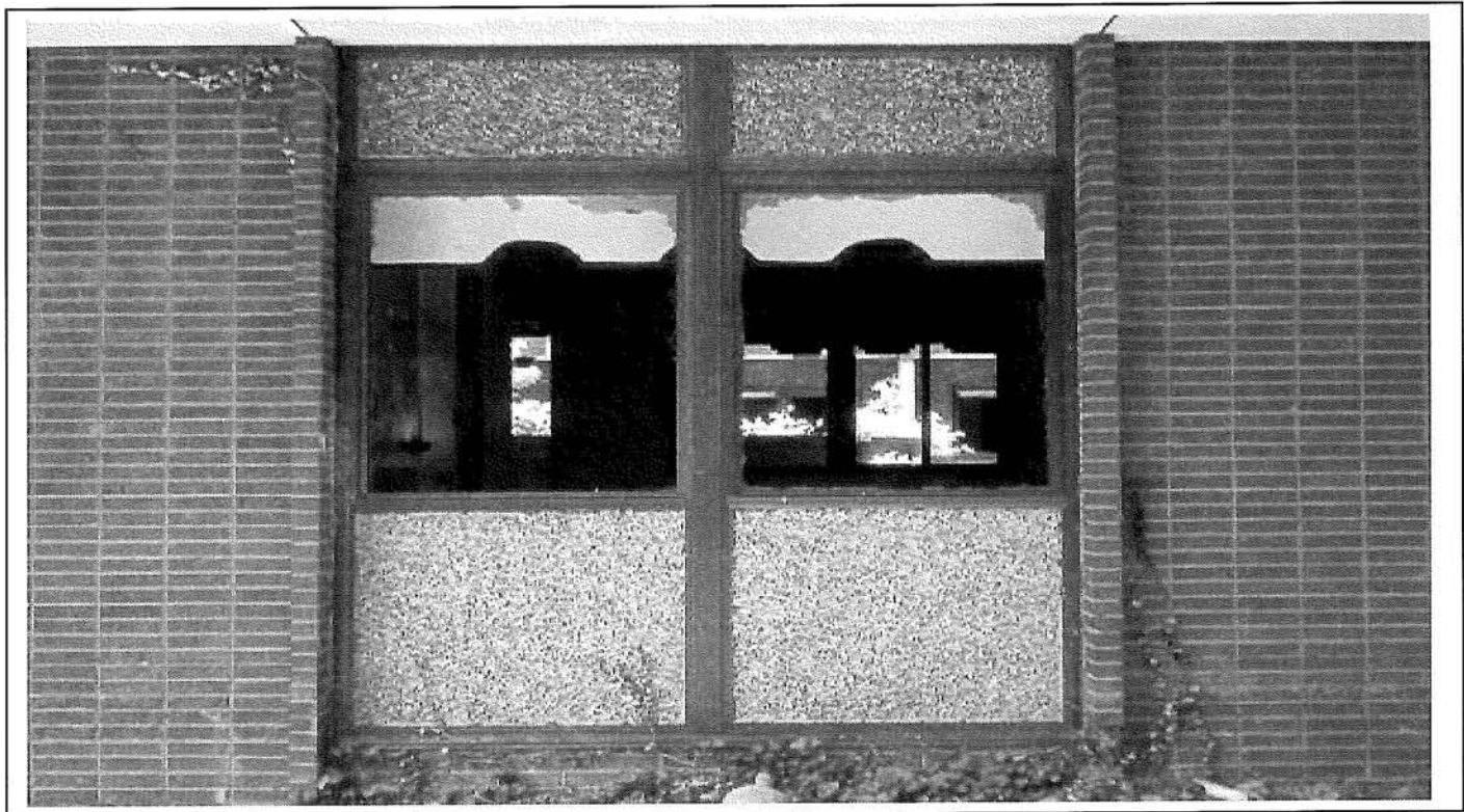
Photo 12: View of the side elevation if cottage No. 3 depicting the metal window framing and aggregate panels.
