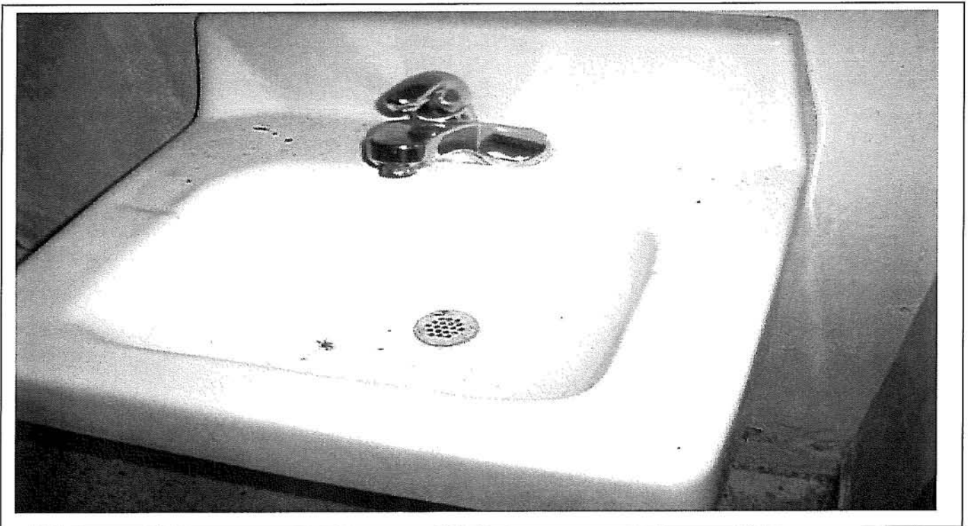
Photo 6: Typical sink with undercoating containing ACM.
