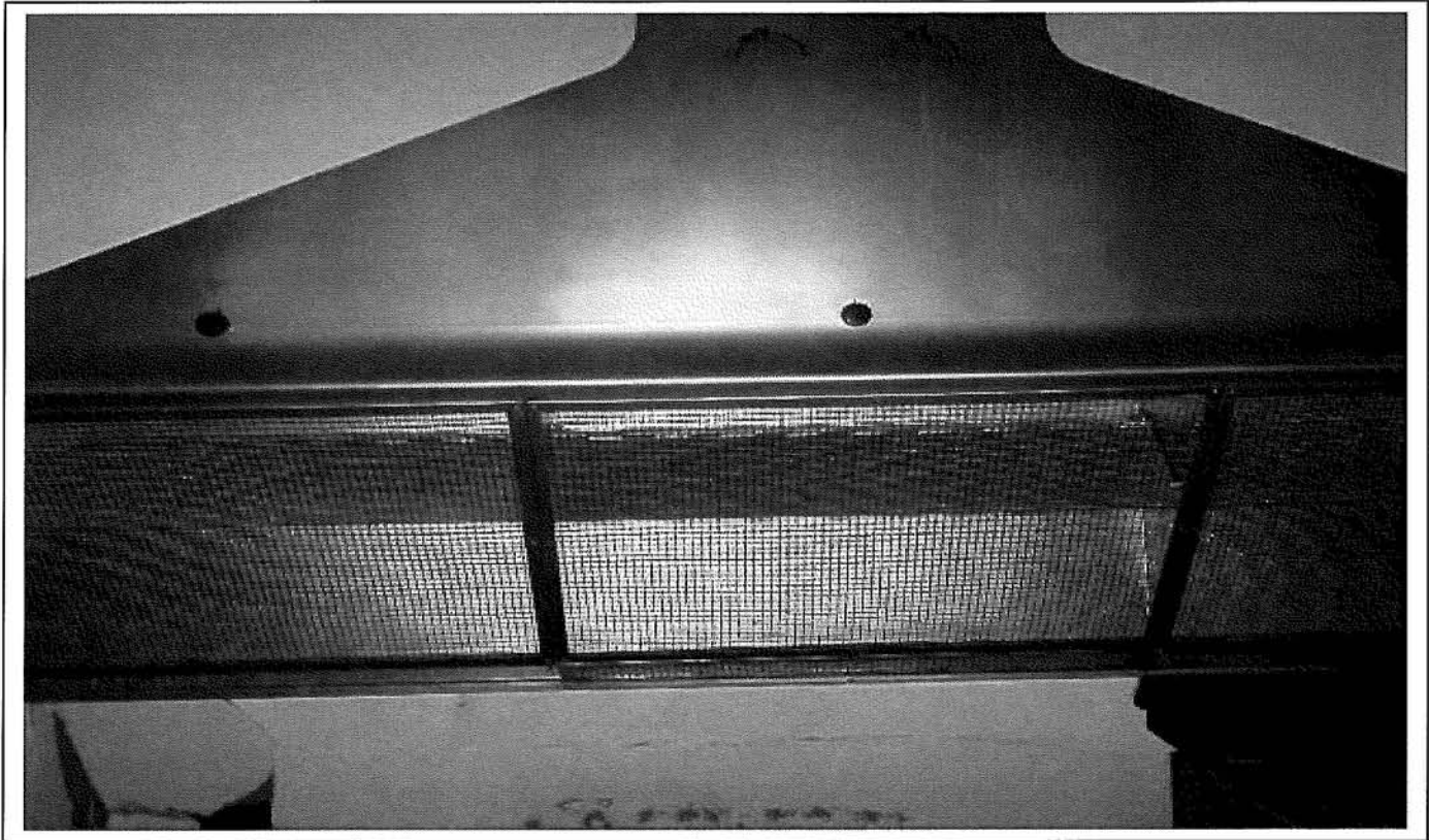
Photo 139: Wall-mounted stainless steel fence head located in the Lab area, second floor, section 5, Therapy building.
