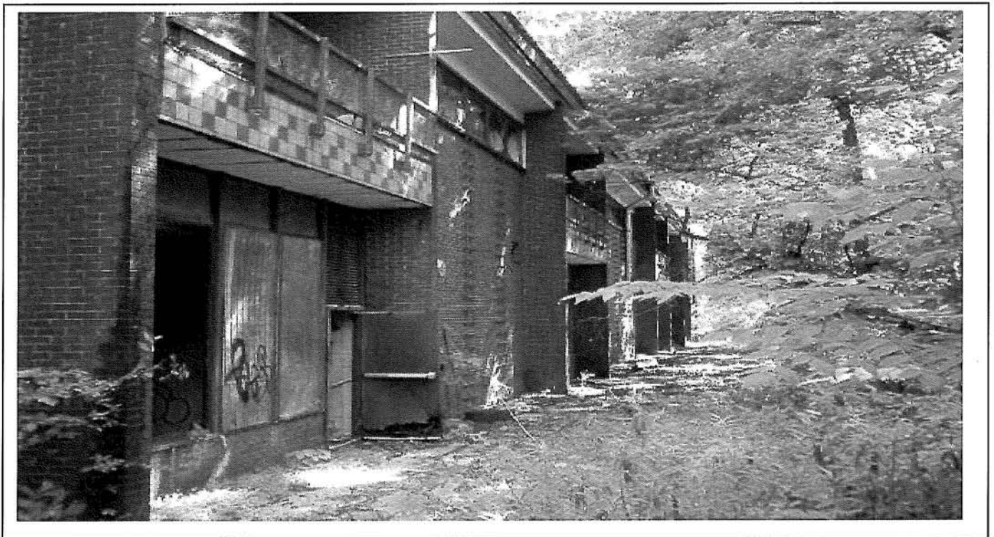
Photo 102: Typical view of rear of Therapy building depicting metal doors & frame, metal railing and Aluminum window frames.
