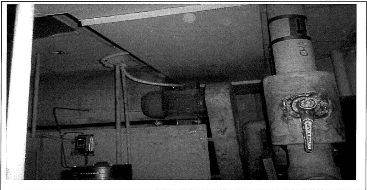
Photo 104: Typical electric motor located in mechanical room in section 4 of Therapy building.
