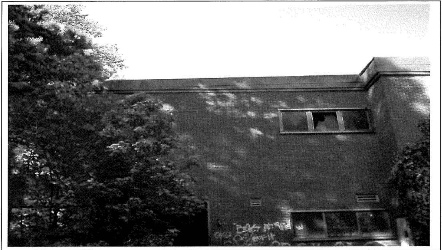
Photo 109: Typical view of metal fascia located around roof perimeter, section 1 of Therapy building.
