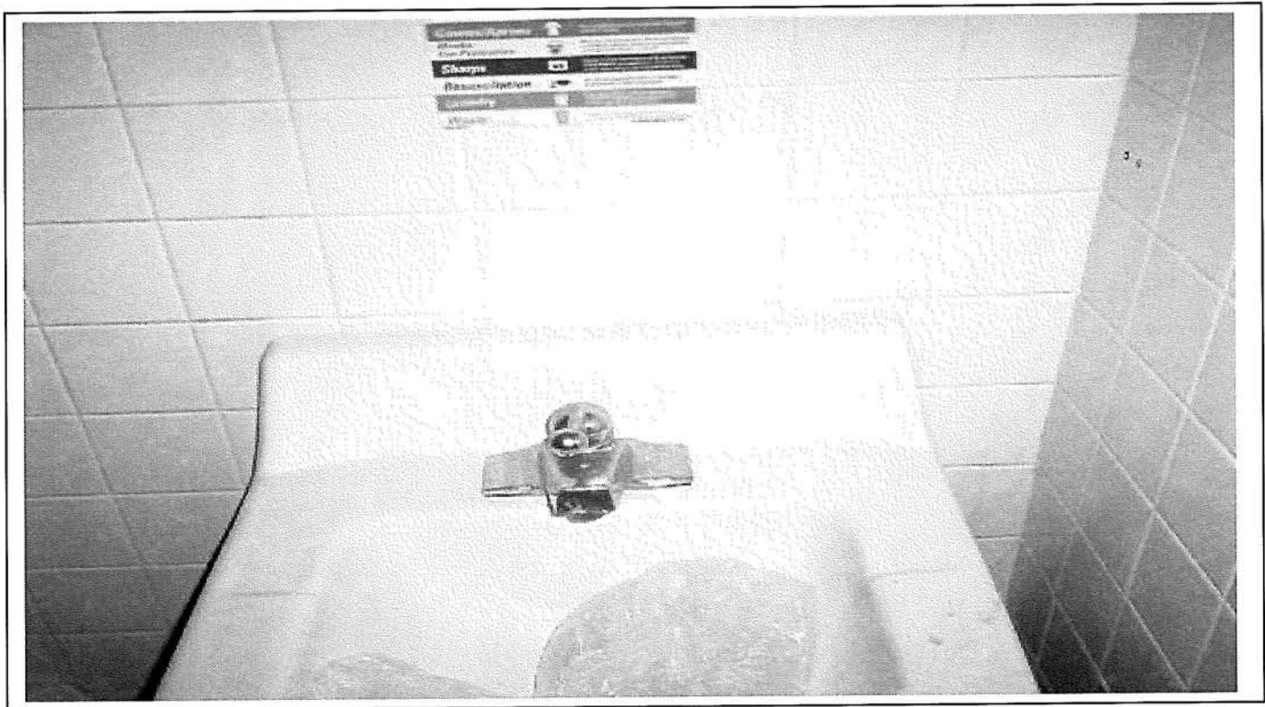
Photo 16: Typical fixtures located in cottages 3, 4, & 5.
