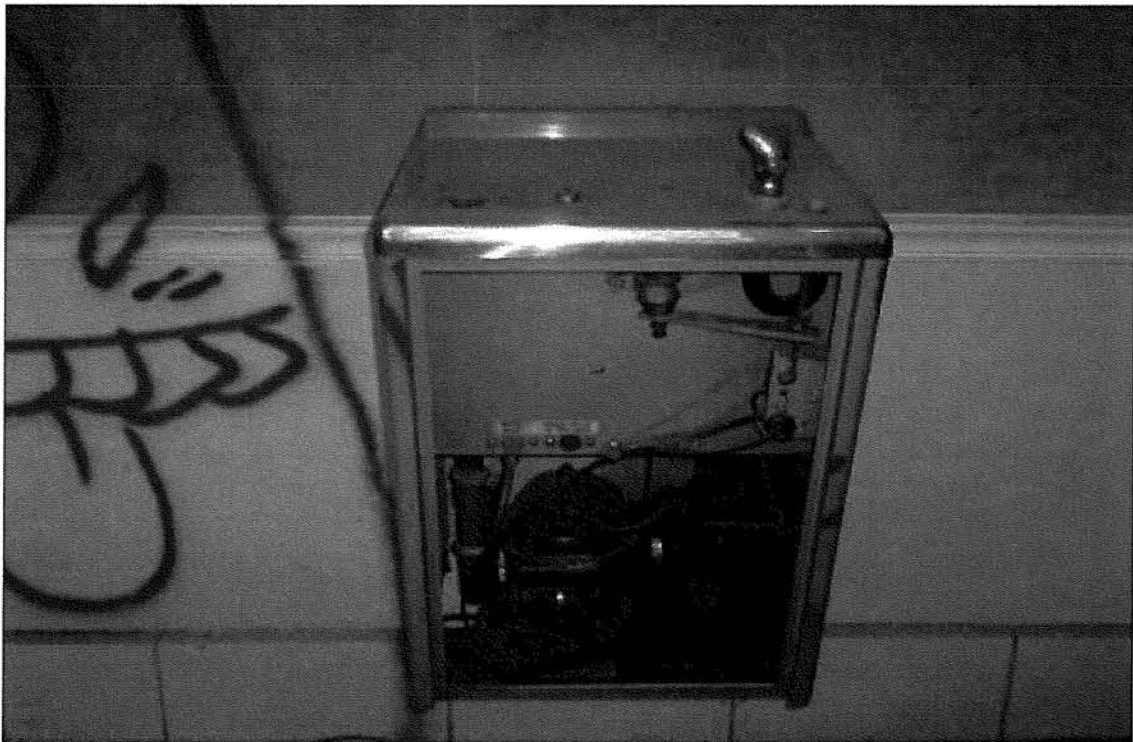
Photo 98: Typical wall-mounted water cooler (fountain) depicting copper elements, located on the ground floor, section 4 Therapy building.
