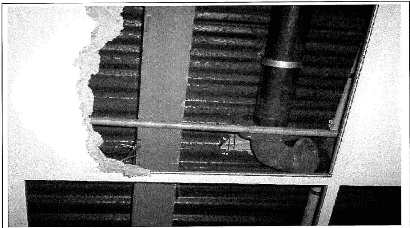
Photo 20: Typical view of section above ceiling in cottage No. 4 depicting structural steel and metal pipes.
