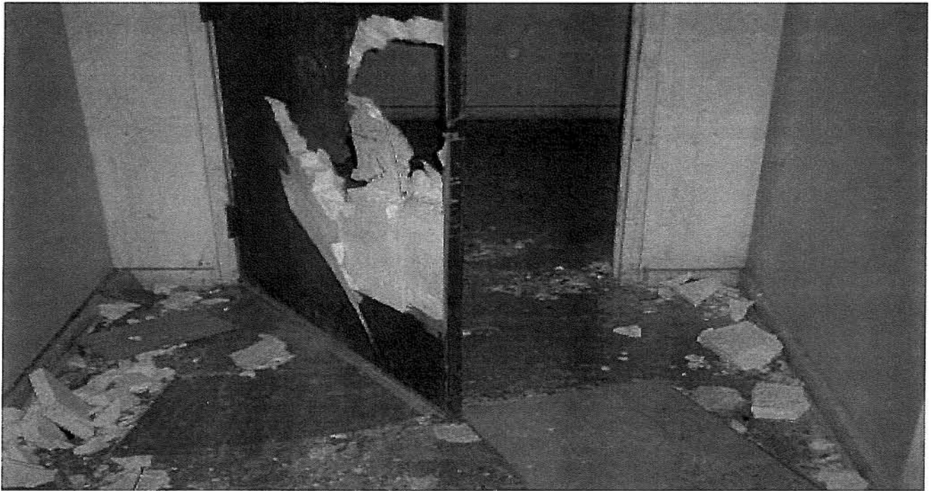
Photo 12: Typical Fire Door with Insulation containing ACM scattered on the floor.
