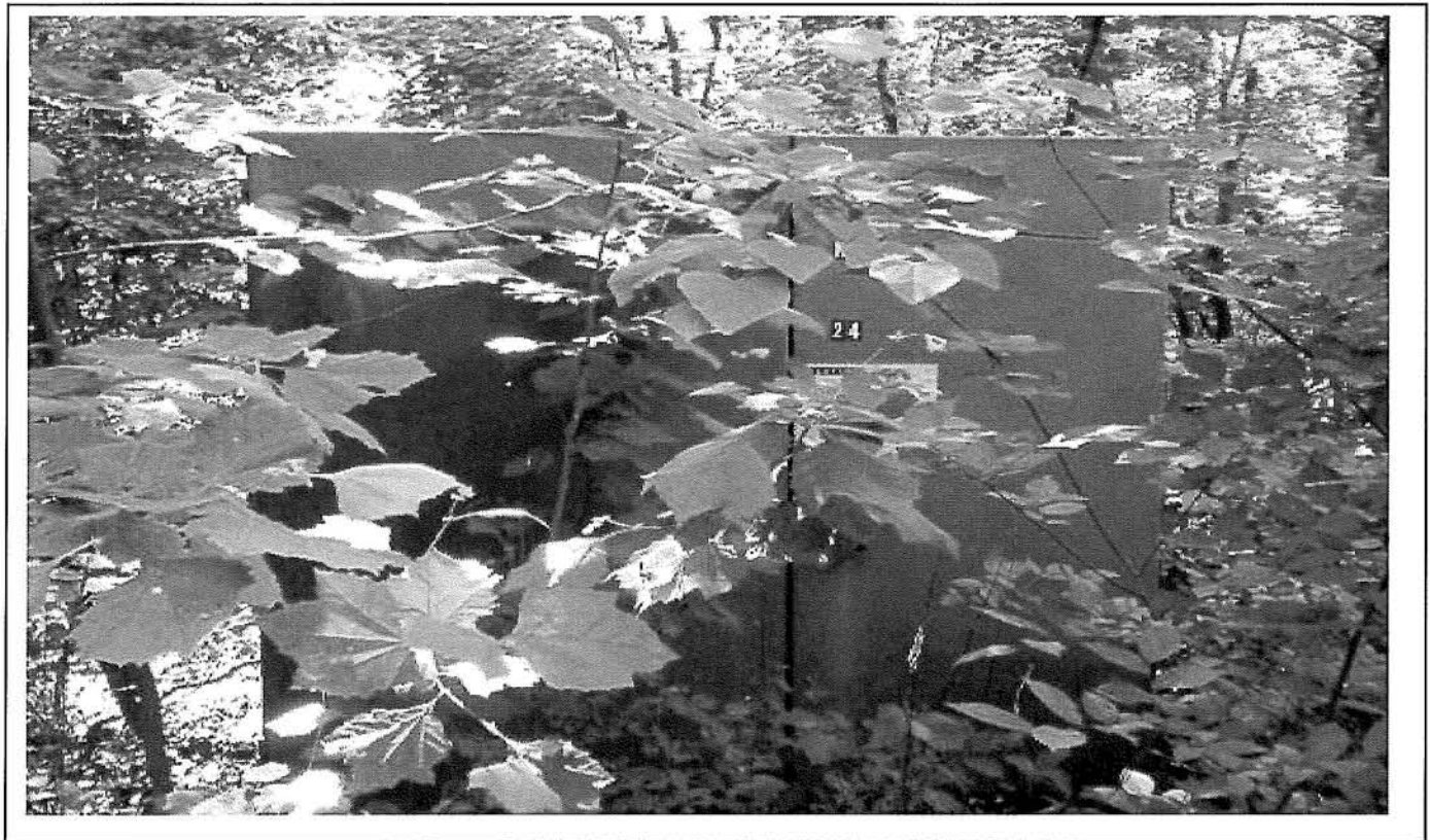
Photo 103: Typical metal transformer case.
