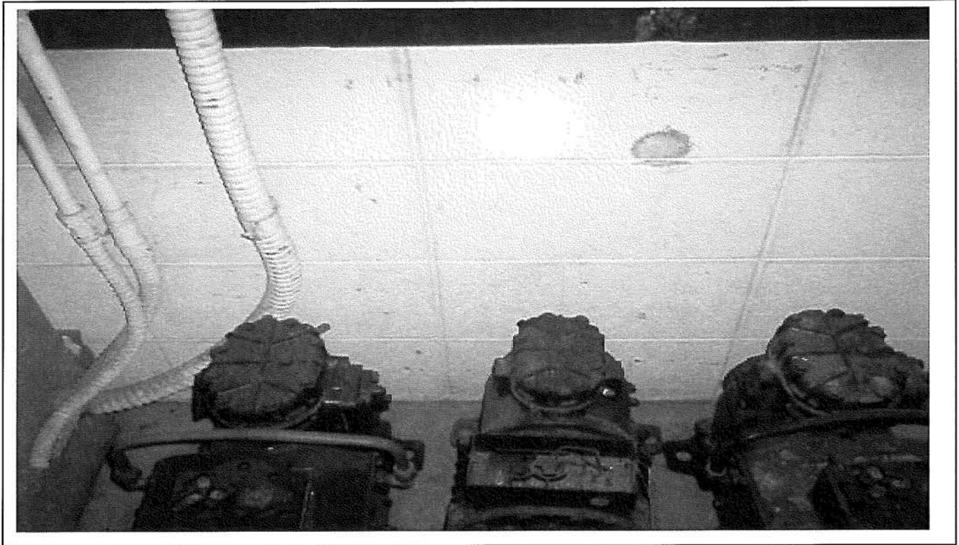
Photo 80: Typical electrical motors stored in mechanical room of section 6, Therapy Building.
