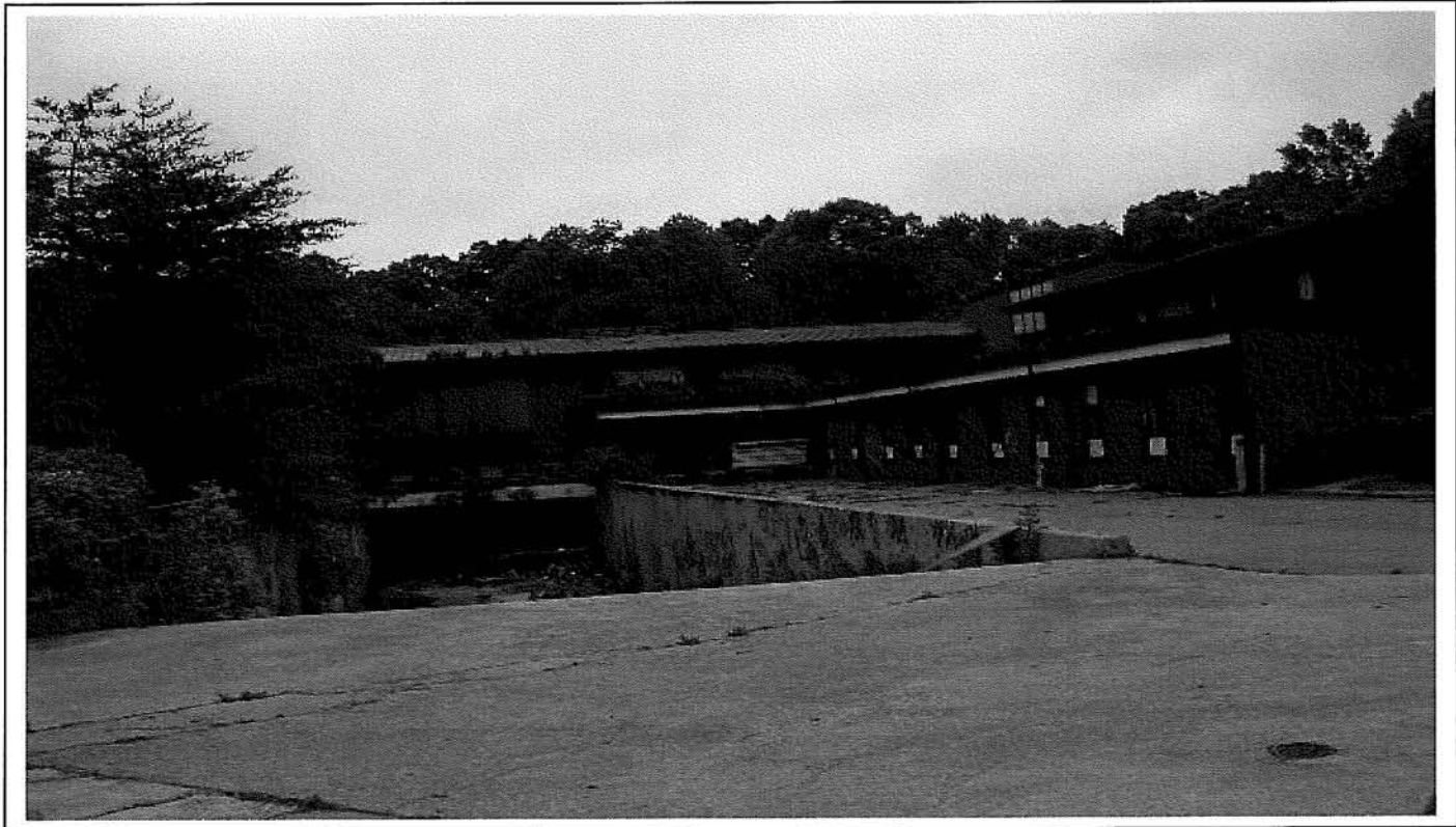
Photo 69: General exterior perspective of the concrete ramp and retaining walls leading to level 2 of the Therapy Building.
