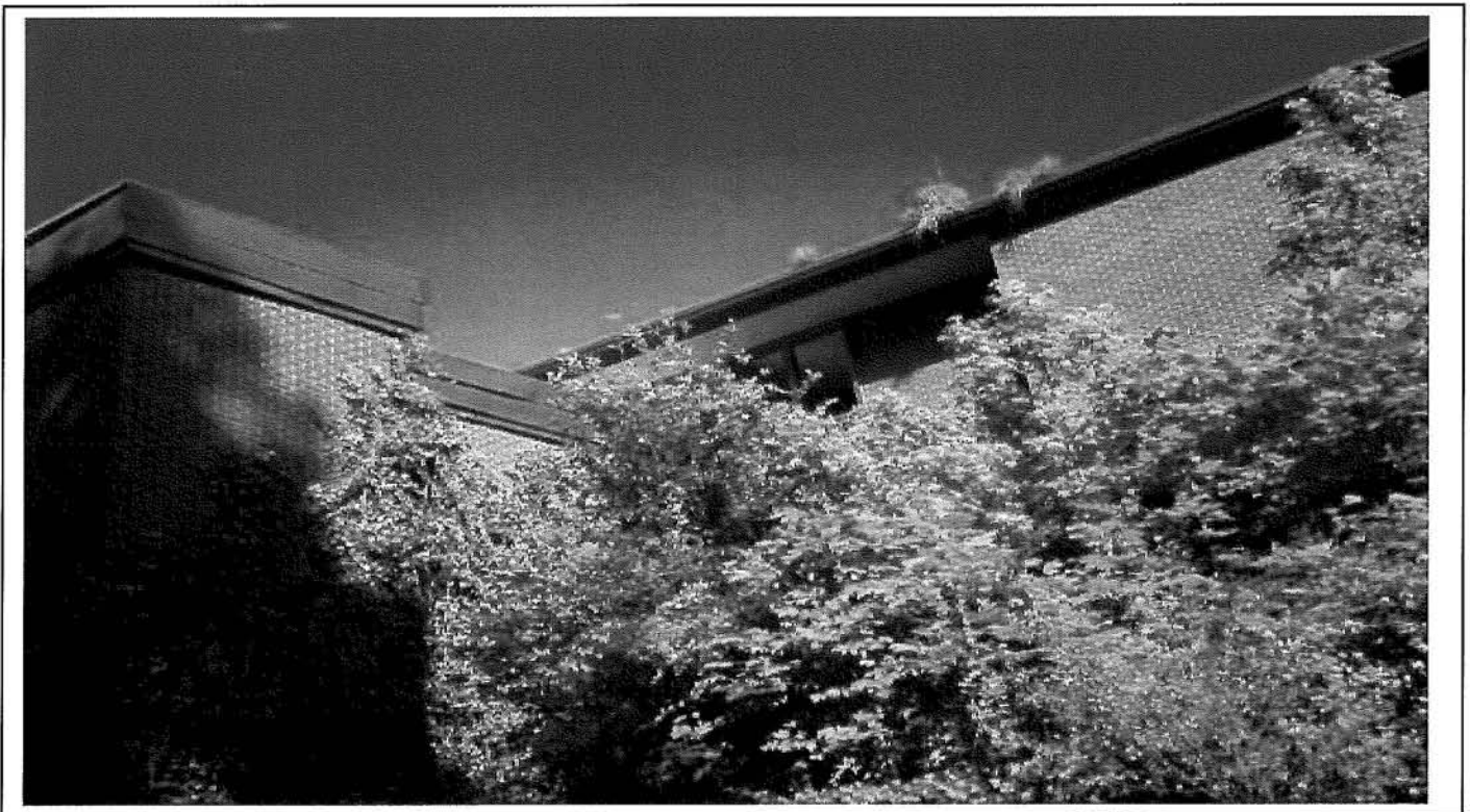
Photo 110: Typical view of metal fascia located around roof perimeter, section 1 of Therapy building.
