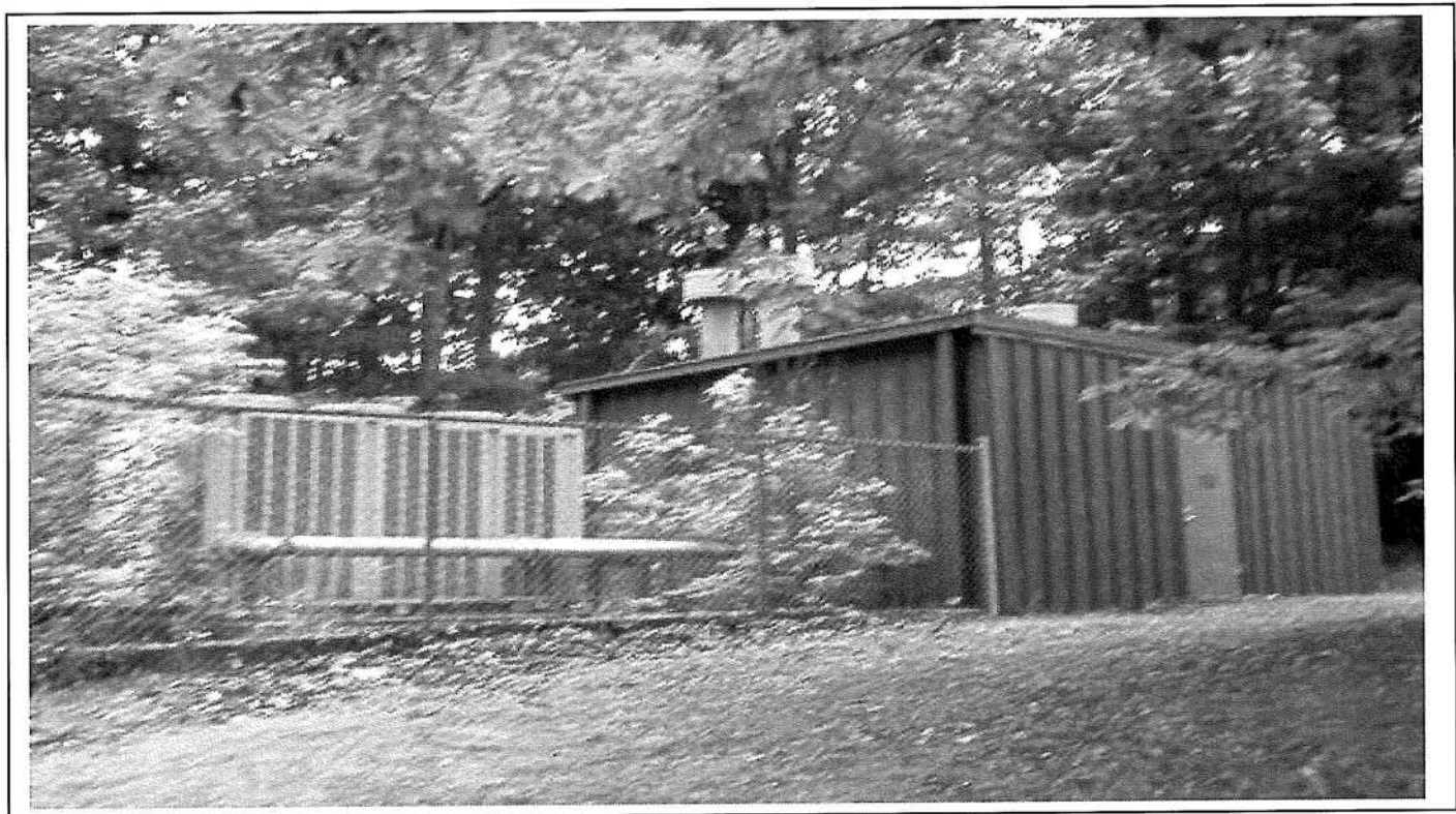
Photo 22: View of electrical equipment building associated with cottage No 4.
