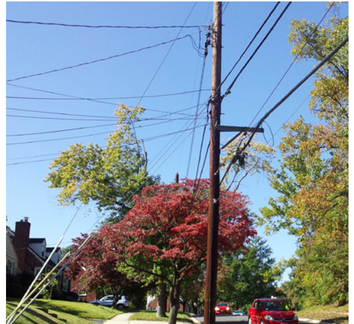
FIGURE 20: EXAMPLE OF EXTENSION ARM ON POLE, ENABLING HORIZONTAL EXPANSION OF CAPACITY
