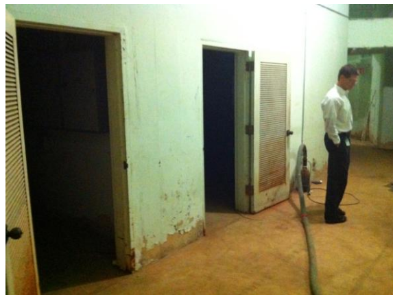
Damaged Wall at Basement
