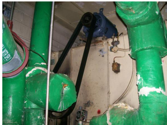
Air Handling Unit
