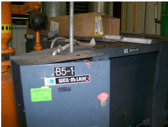
Gas-Fired Hydronic Boiler
