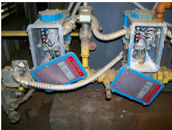
Boiler Burner Controls
