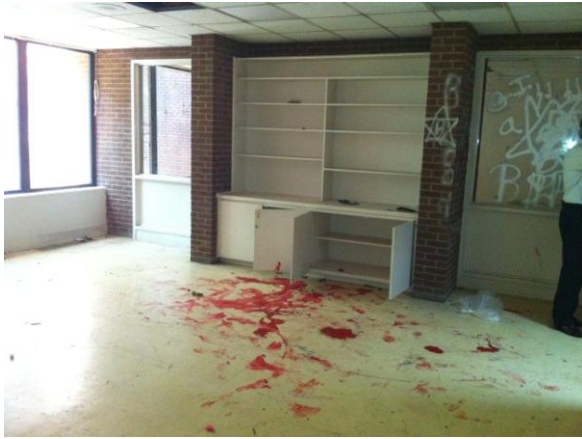
Vandalism at Classroom
