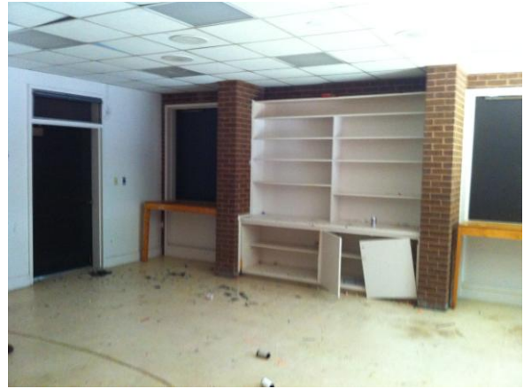
Damaged Flooring & Millwork
