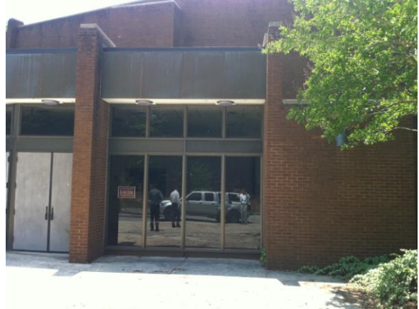
Original Glazing in Aluminum Storefront
