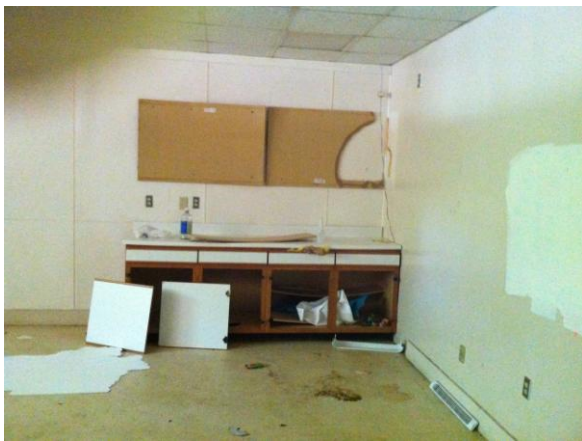
Damaged Flooring & Millwork
