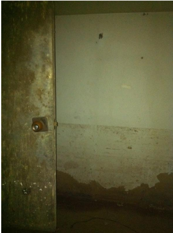
Deteriorated Basement Door & Hardware
