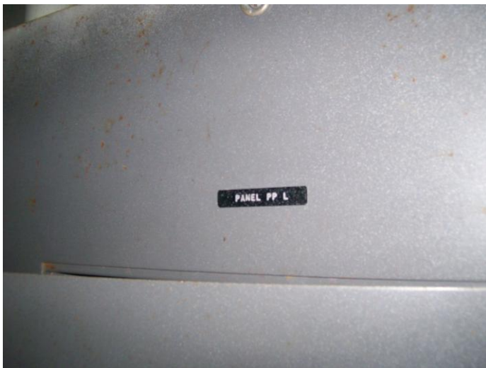
Main Distribution Panel "PP-L"
