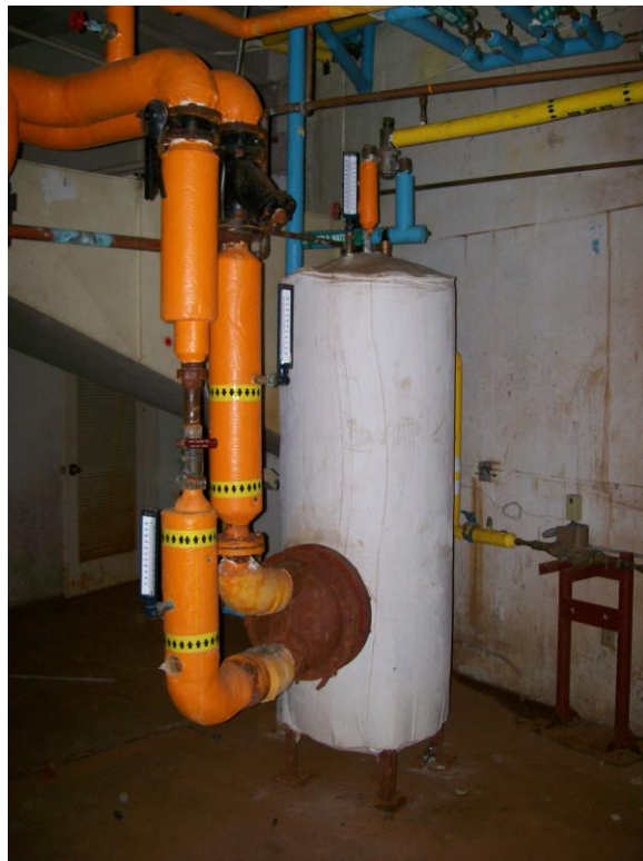
Domestic Water Heat Exchanger
