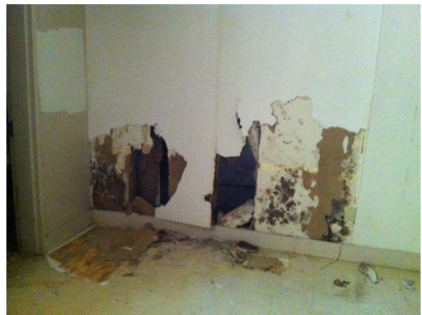
Water Damage & Mold at Wall
