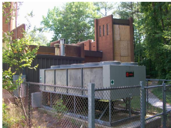
Chiller at Rear of Facility
