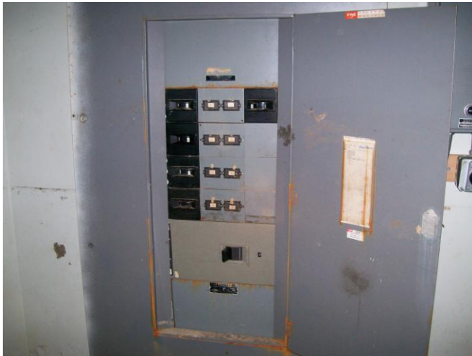
Water Damage at Main Distribution Panel "PP-L"
