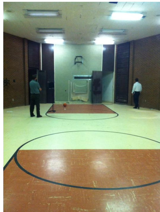
Damaged Walls at Recreation Room
