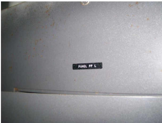
Main Distribution Panel "PP-L"
