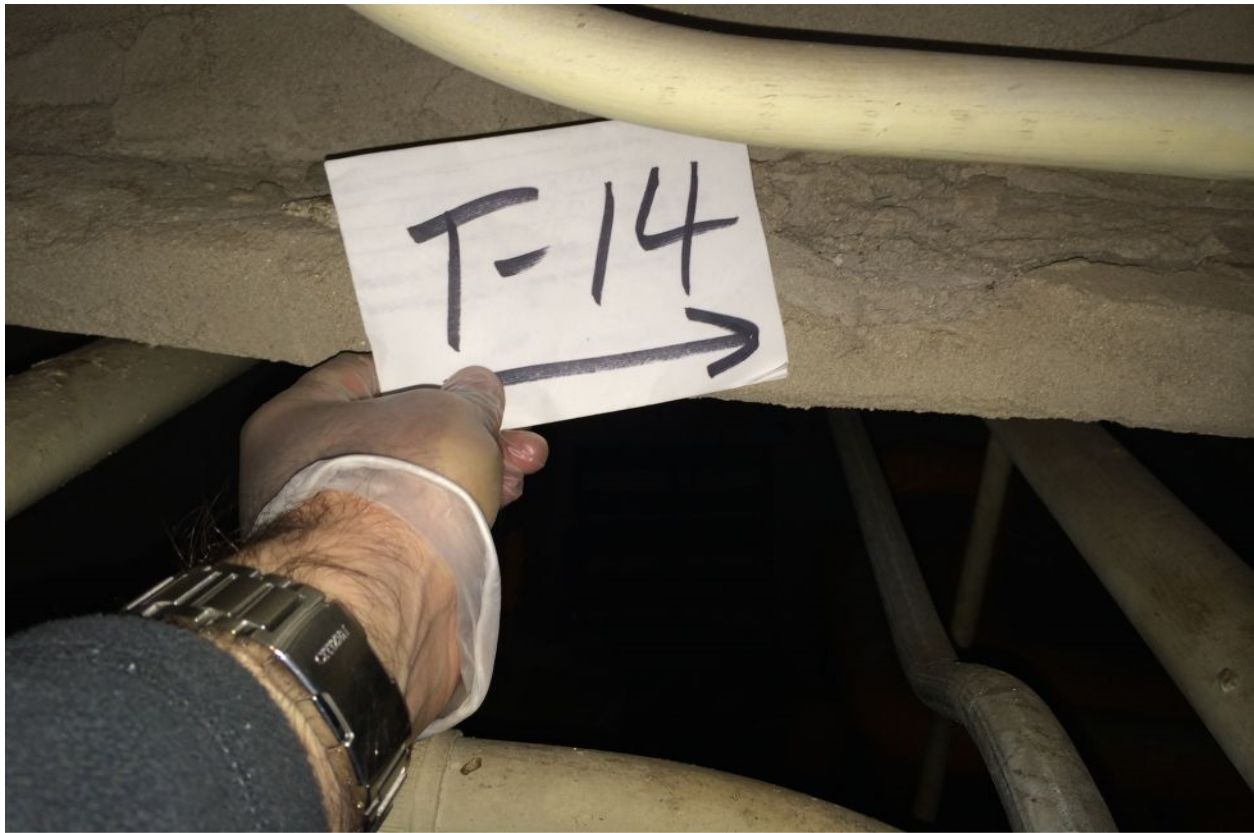
Plate 65: Laboratory analyses detected 20% chrysotile asbestos within spray on surfacing material sample TS-14 collected from the Theatre Building basement structural steel.
