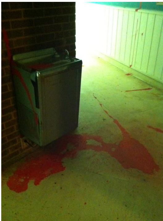
Vandalism at Corridor
