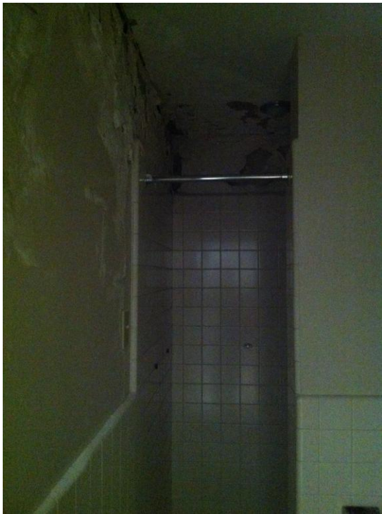
Damaged Wall at Restroom/Shower
