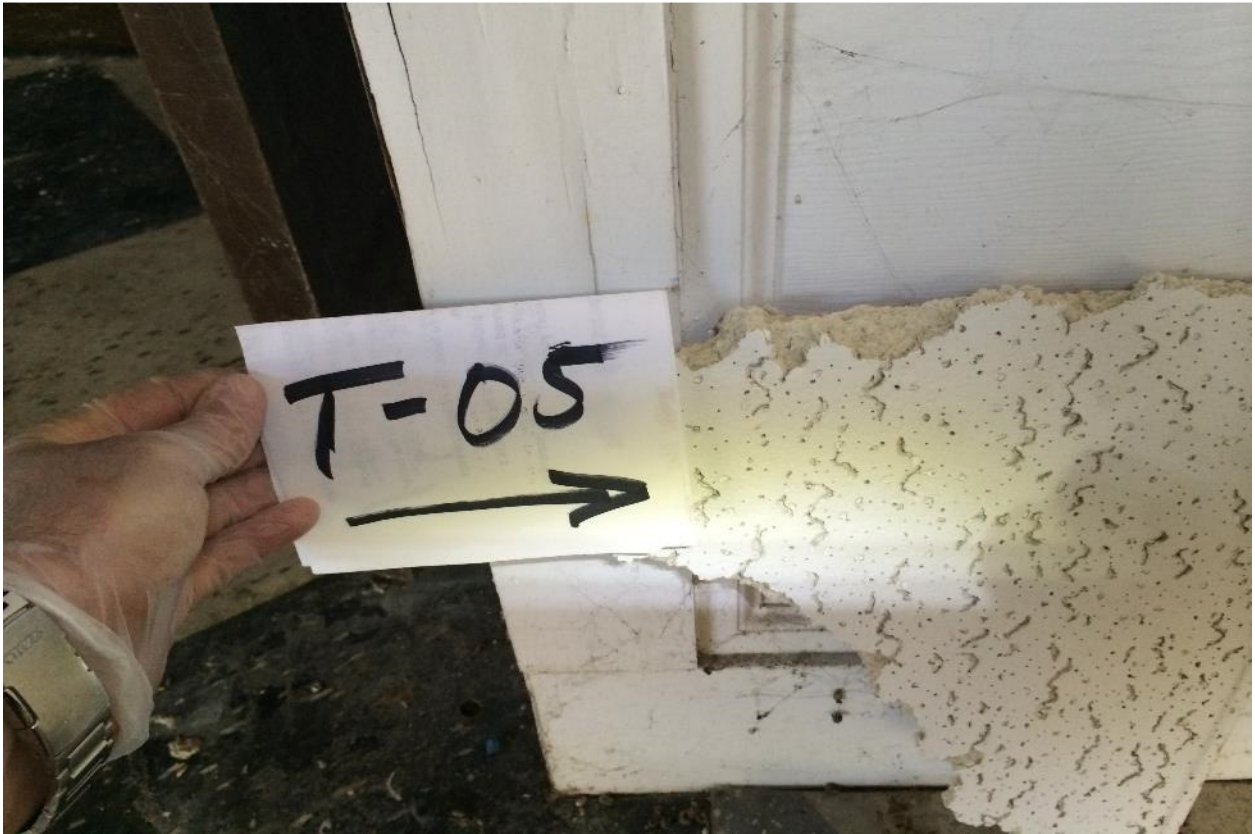
Plate 56: Laboratory analyses detected 2% chrysotile asbestos within suspended ceiling tile sample TS-05 collected from the Theatre Building lobby area.
