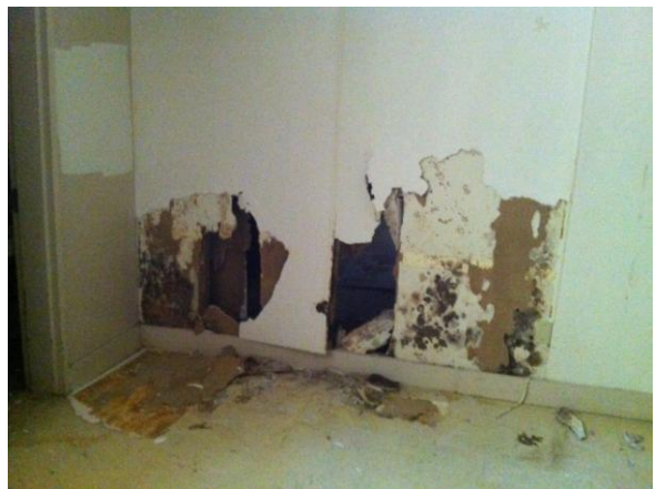
Water Damage & Mold at Wall
