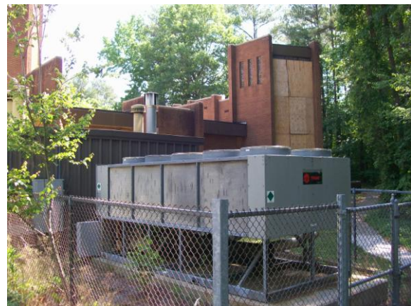
Chiller at Rear of Facility
