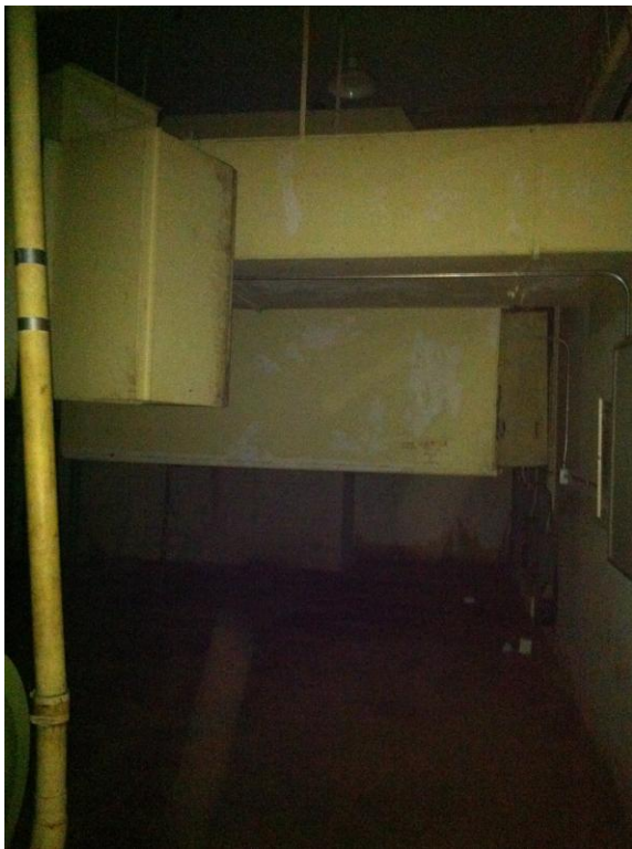
Ductwork in Basement
