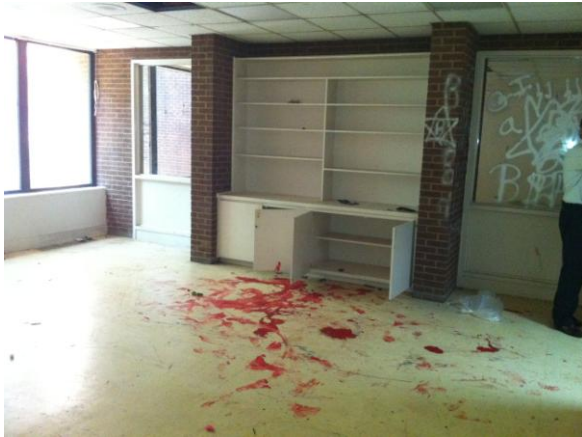
Vandalism at Classroom
