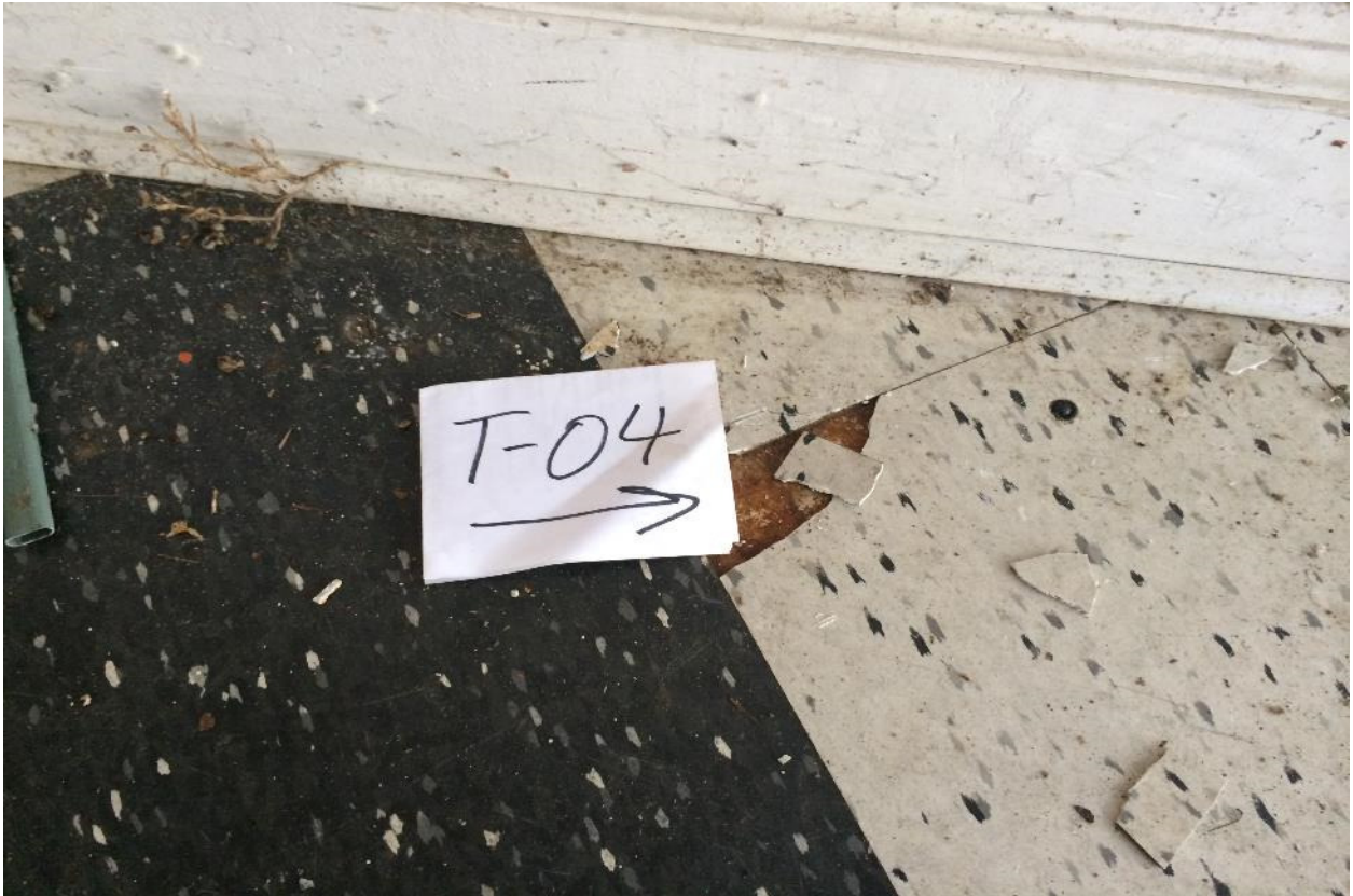
Plate 55: Laboratory analyses did not detect asbestos minerals within the white floor tile from sample TS-04 but did detect 5% chrysotile asbestos in the mastic from sample TS-04 collected from the Theatre Building lobby area.
