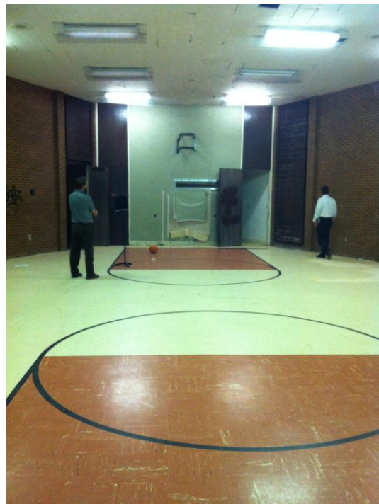
Damaged Walls at Recreation Room
