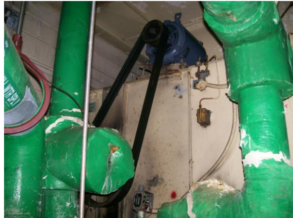
Air Handling Unit
