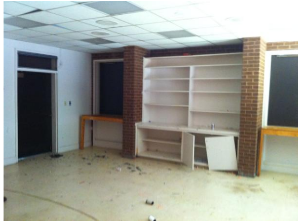
Damaged Flooring & Millwork
