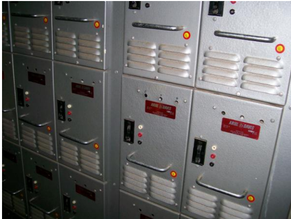
Theater Dimmer Module Control Center
