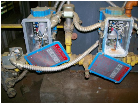
Boiler Burner Controls
