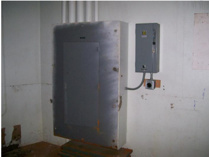
Water Damage at Main Distribution Panel "PP-L"
