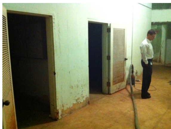
Damaged Wall at Basement
