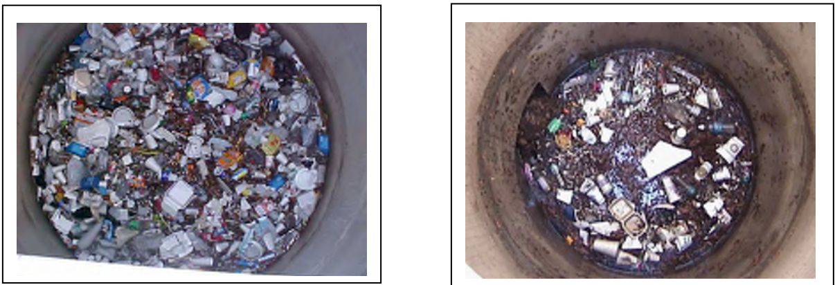
Figure 20 Gross Pollutants Captured in the CDS Units Sump
