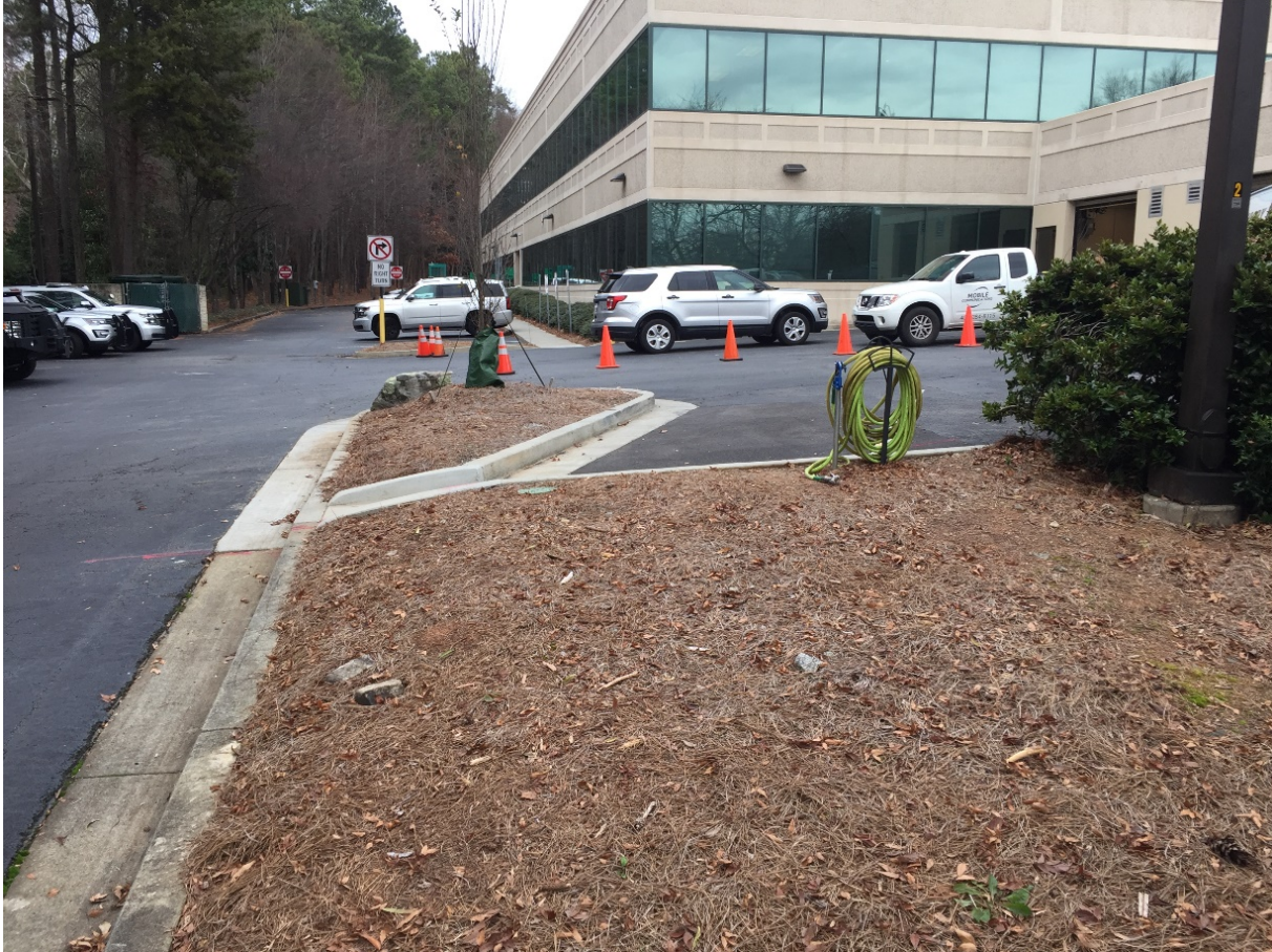
Landscaped island location of underground oil-grit separator unit
