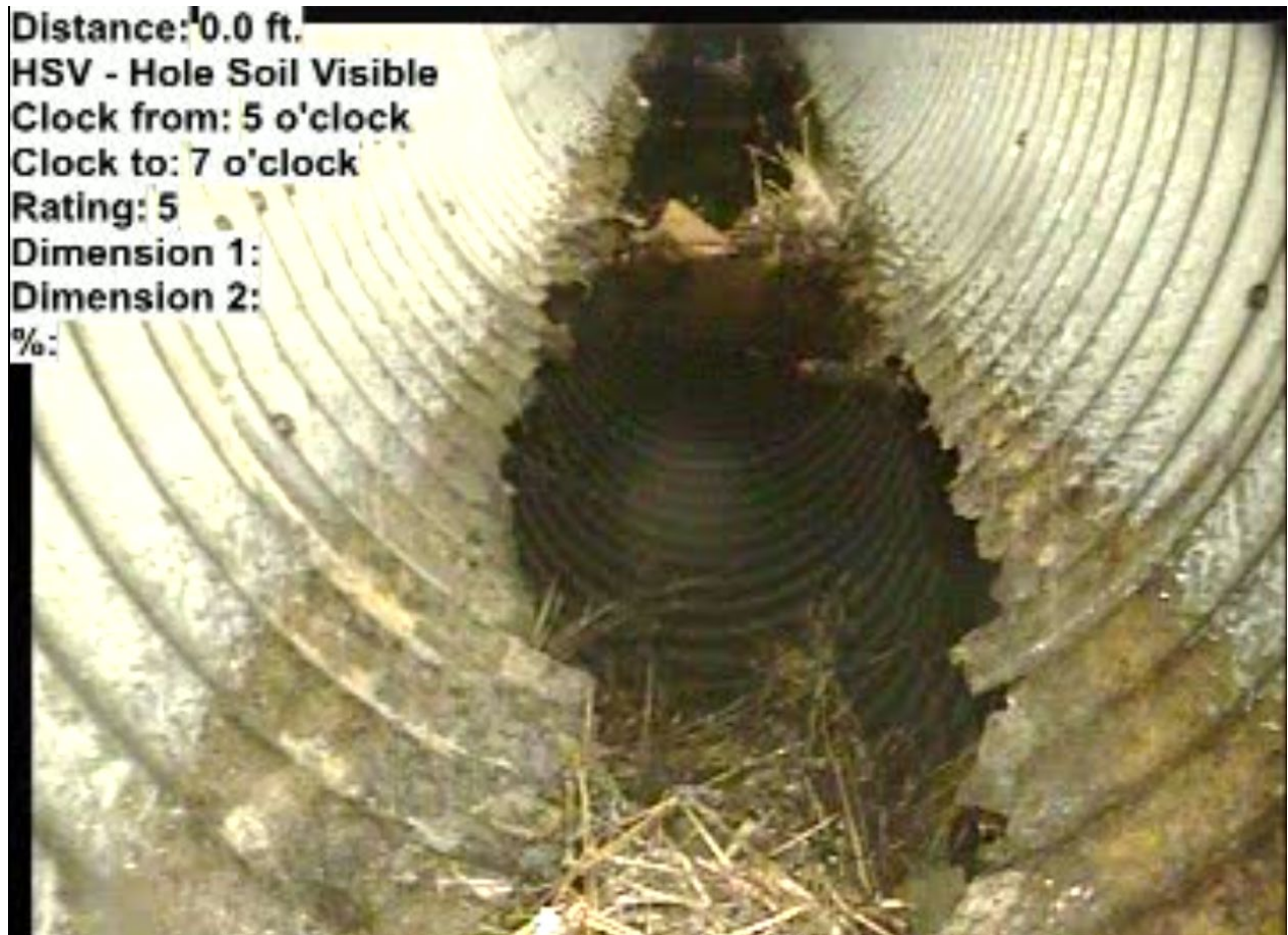
Severe Corrosion with Visible Holes
