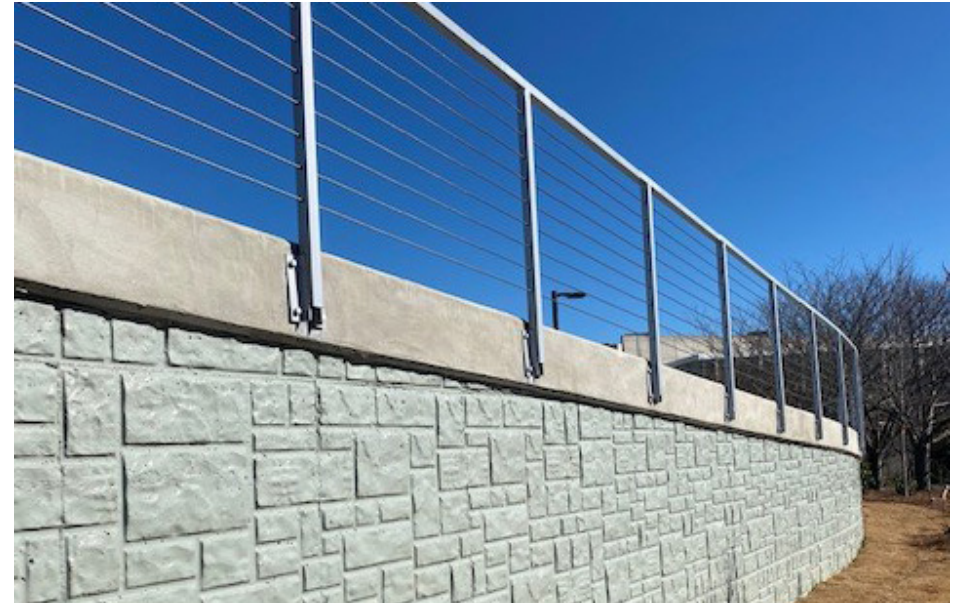
Post and cable railing provides a safe trail edge while acting as a visually lighter option.
