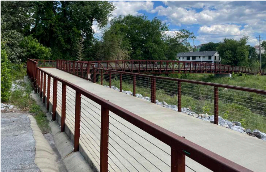
An example of the cable handrail with corten steel posts and top rail.
