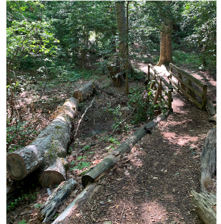
Significant erosion damage and storm damage exists along stream through wooded area adjacent to eco-classroom area.
