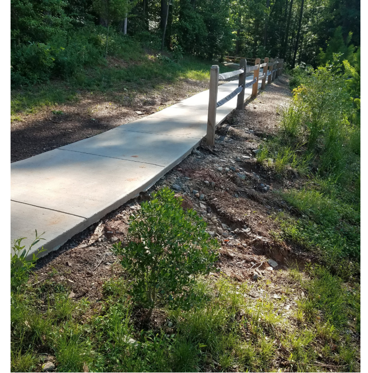
Stormwater runoff is undercutting the existing sidewalk north of the pond, creating a safety hazard.
