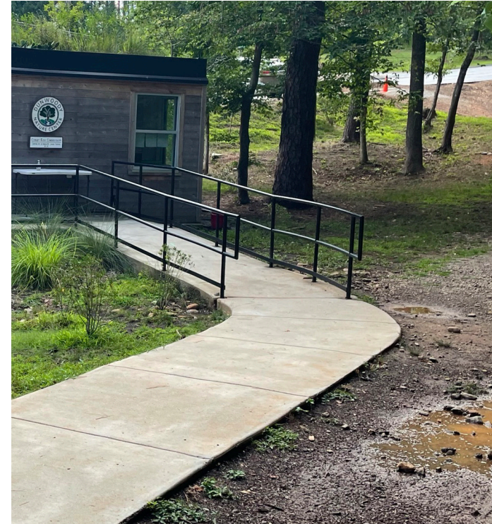
Evidence of stormwater runoff pooling, creating a muddy area around the existing classroom.
