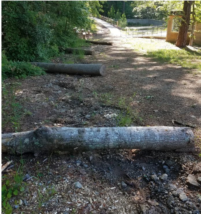
Evidence of erosion upstream of stormwater pond.
