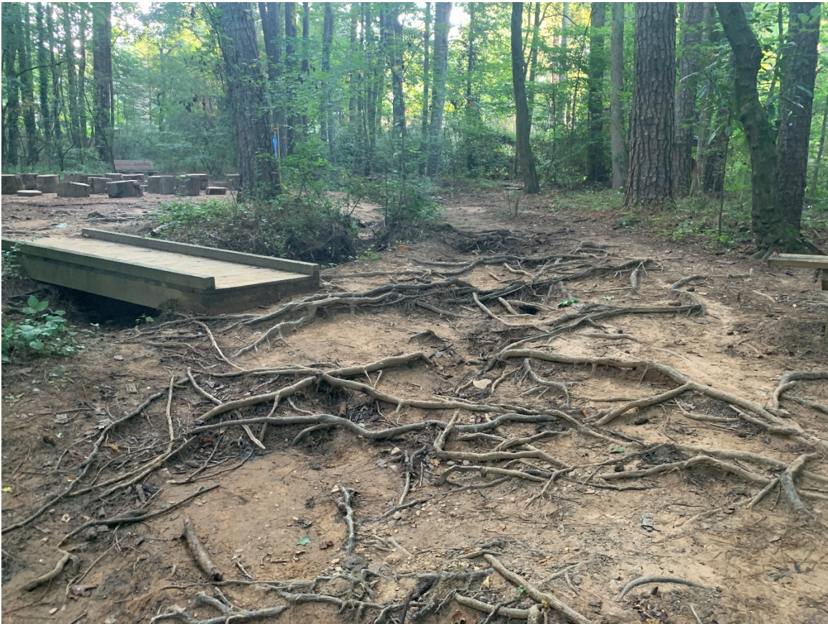
Figure 2 – Active erosion due to pedestrian traffic and overland flow adjacent to wetland
