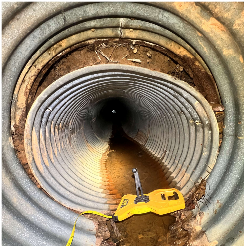
Severe Deformation, Fracture Formation with Exposed Soil and Corrosion
