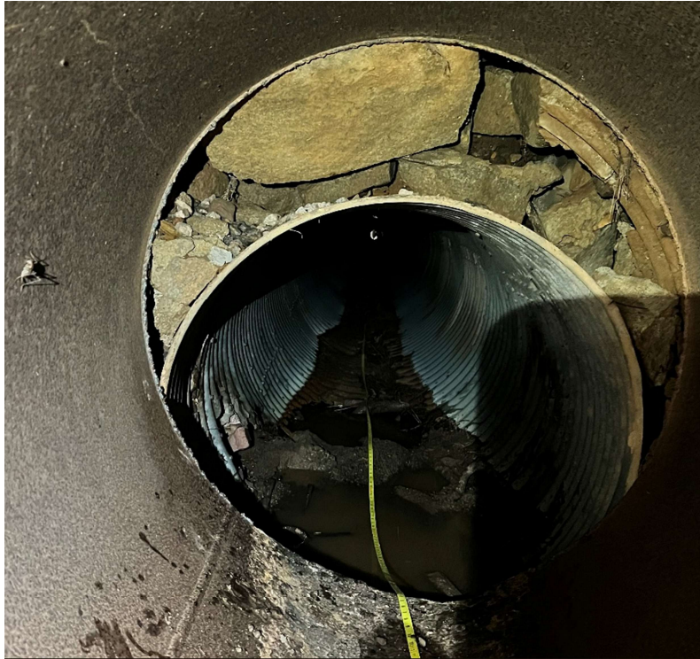
Large Offset at Upstream Joint
